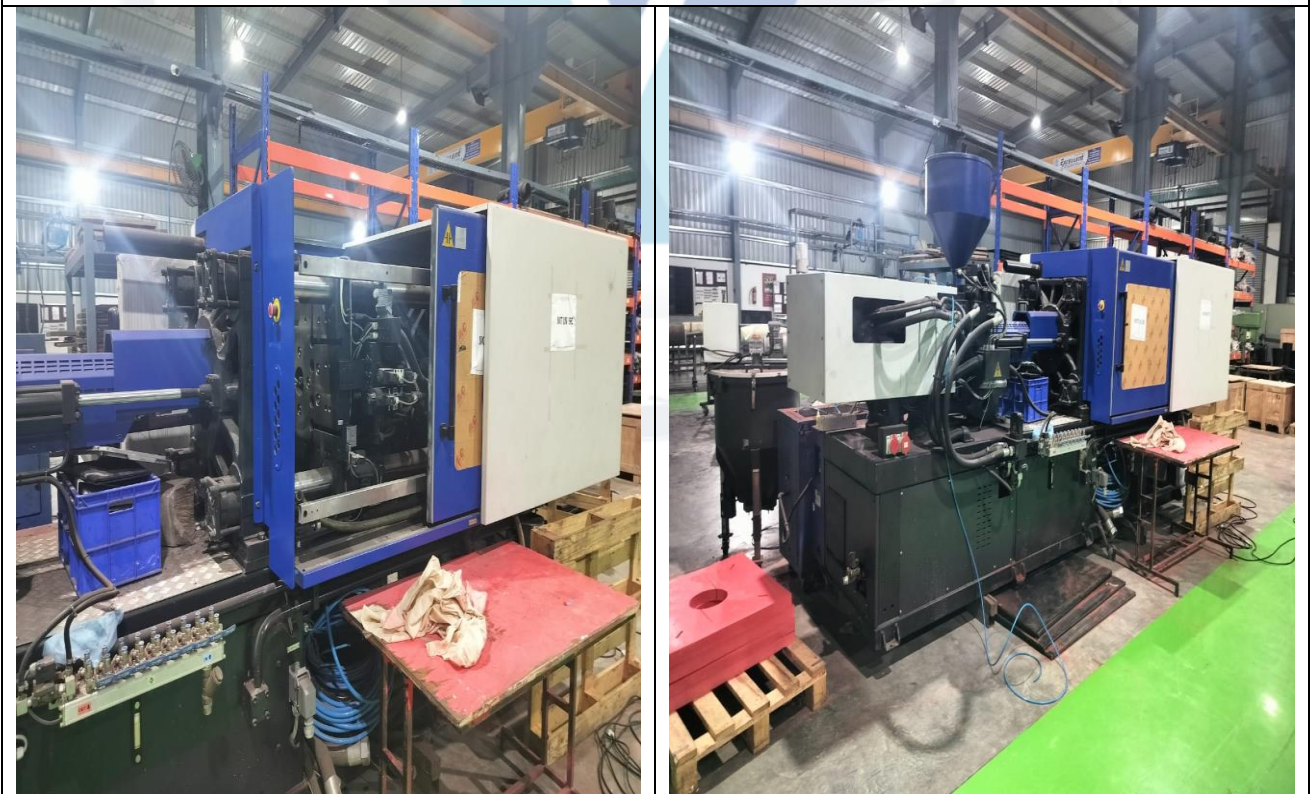
Plastic Injection Moulding Machine MA 2000/770G at Location-2
