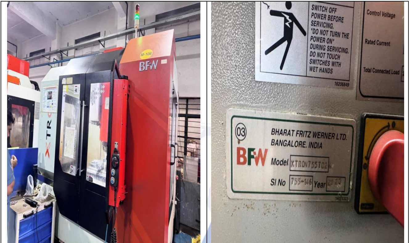
View of CNC Vertical Machining Center Model: Xtron 755 with Mitsubishi M80, Sr. No.755-146 Installed at Unit-3
