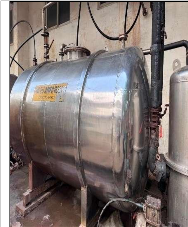
5 KL Horizontal Receiver Tank
