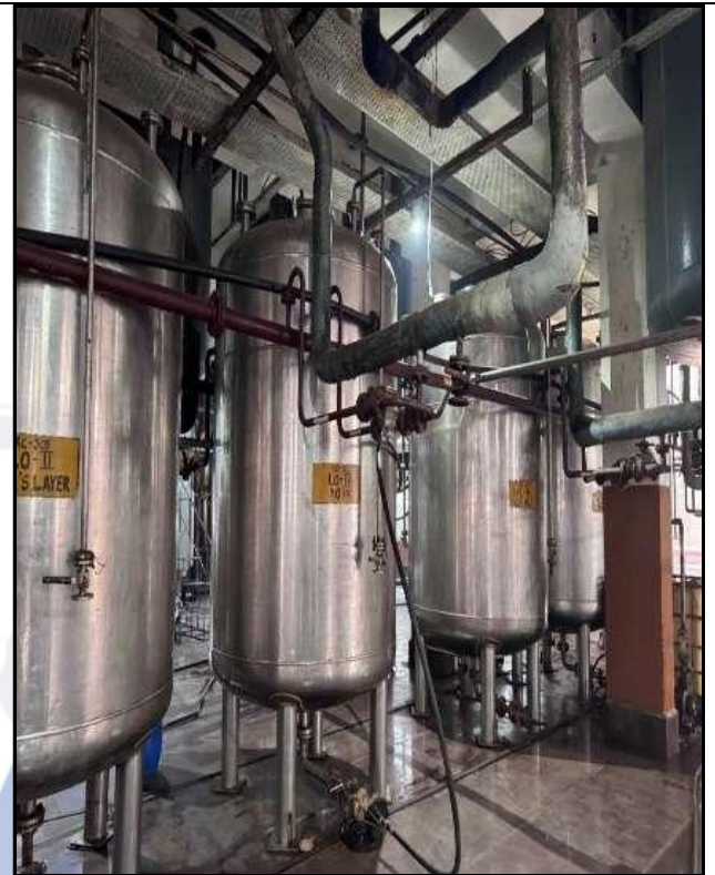
2 KL Receiver Tank
