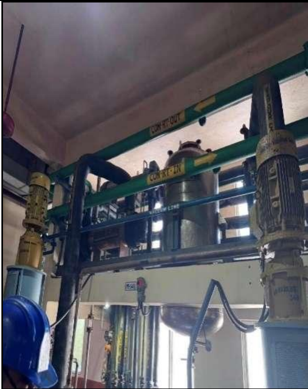
2 KL Receiver Tank
