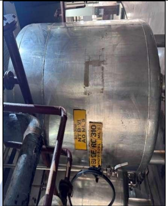
5 KL Receiver Tank
