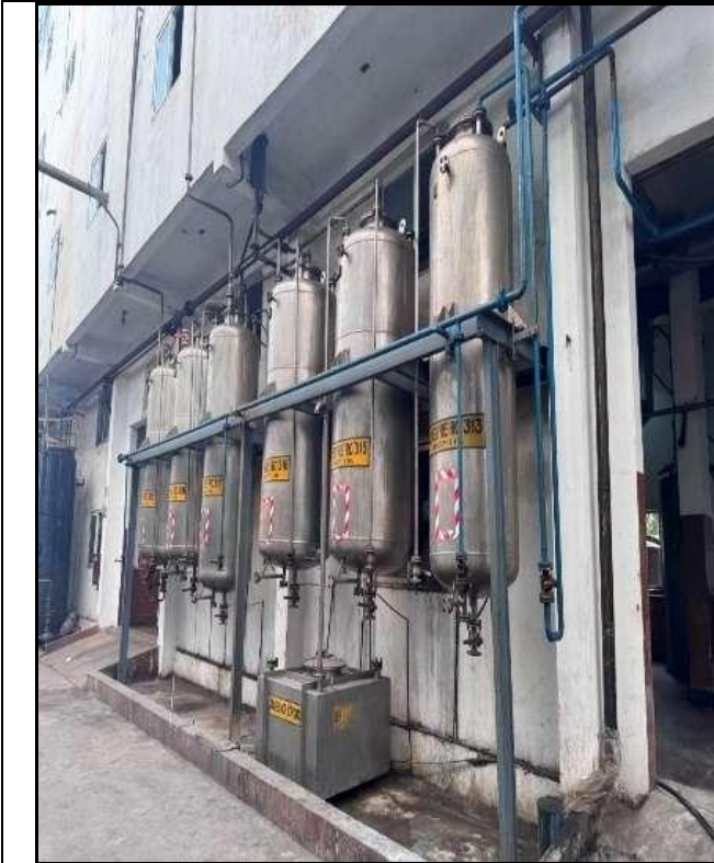
2 KL Receiver Tank
