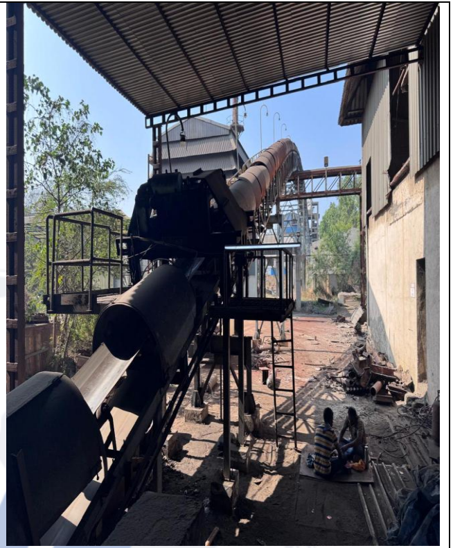
Coal Handling System
