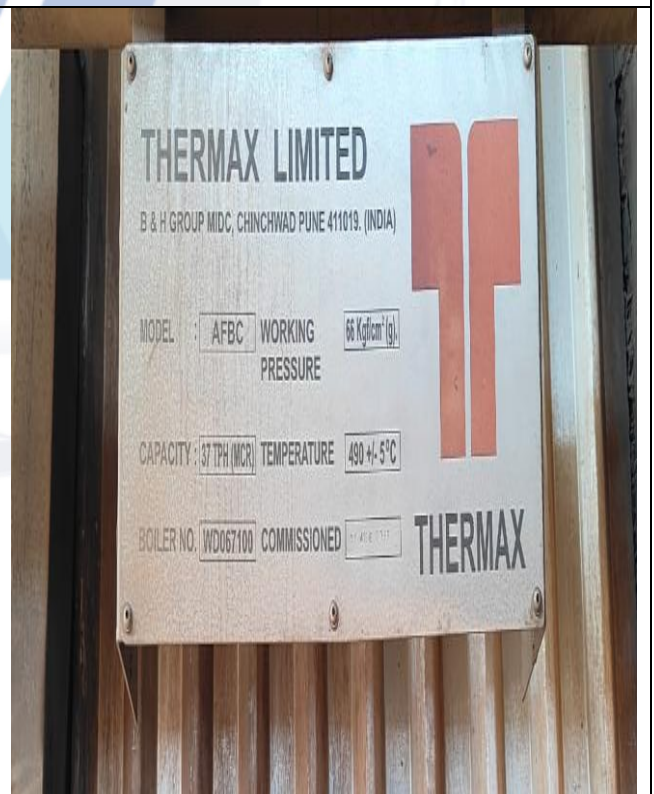
Name Plate of Boiler
