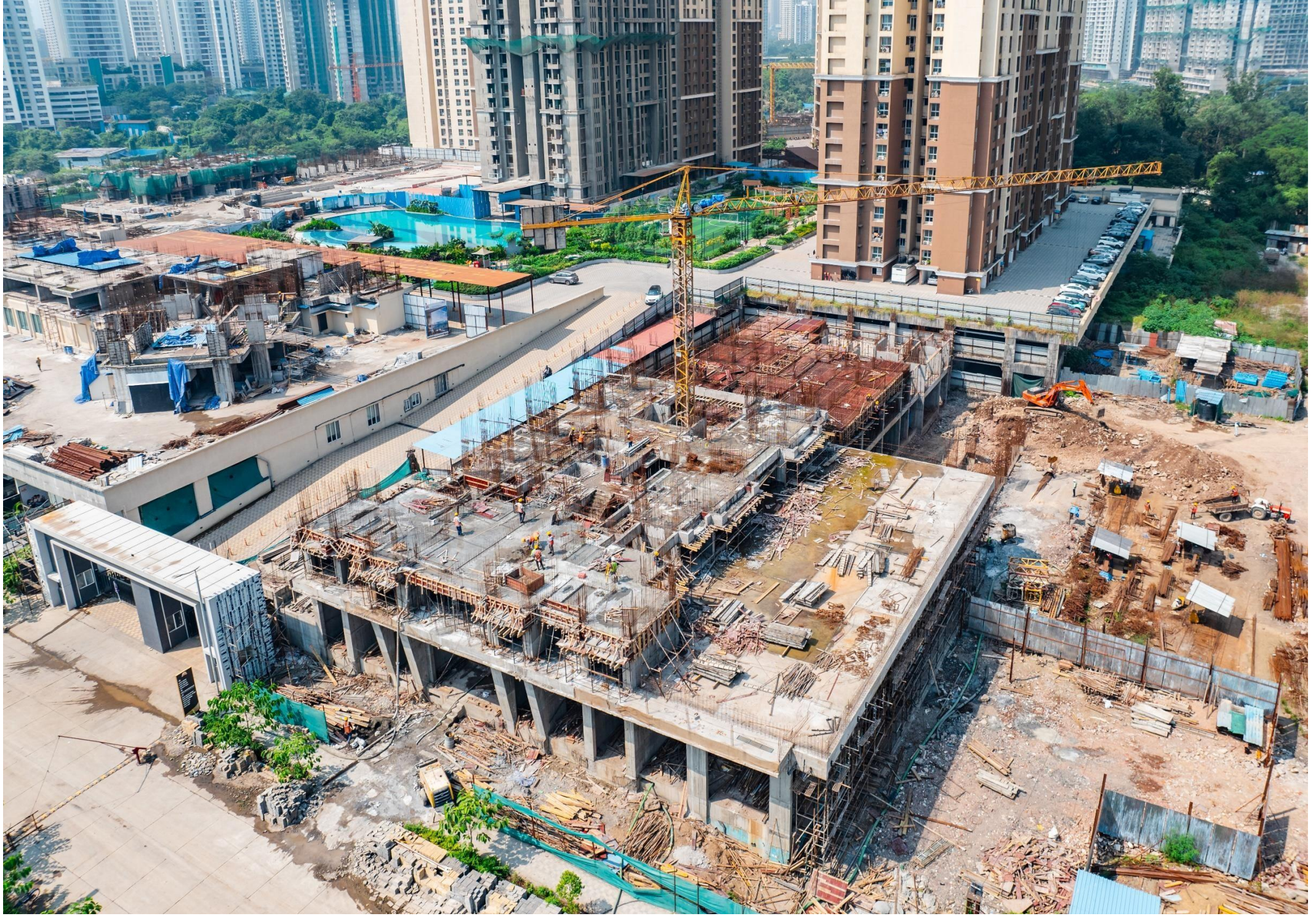
MAPLE A WING - PODIUM FLOOR LEVEL SLAB WORK IN PROGRESS & MAPLE B WING - 1 ST FLOOR LEVEL SLAB WORK COMPLETED
