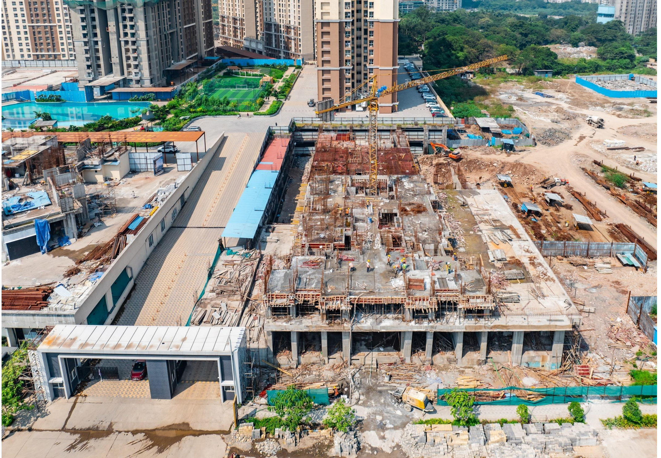
MAPLE A WING - PODIUM FLOOR LEVEL SLAB WORK IN PROGRESS & MAPLE B WING - 1 ST FLOOR LEVEL SLAB WORK COMPLETED
