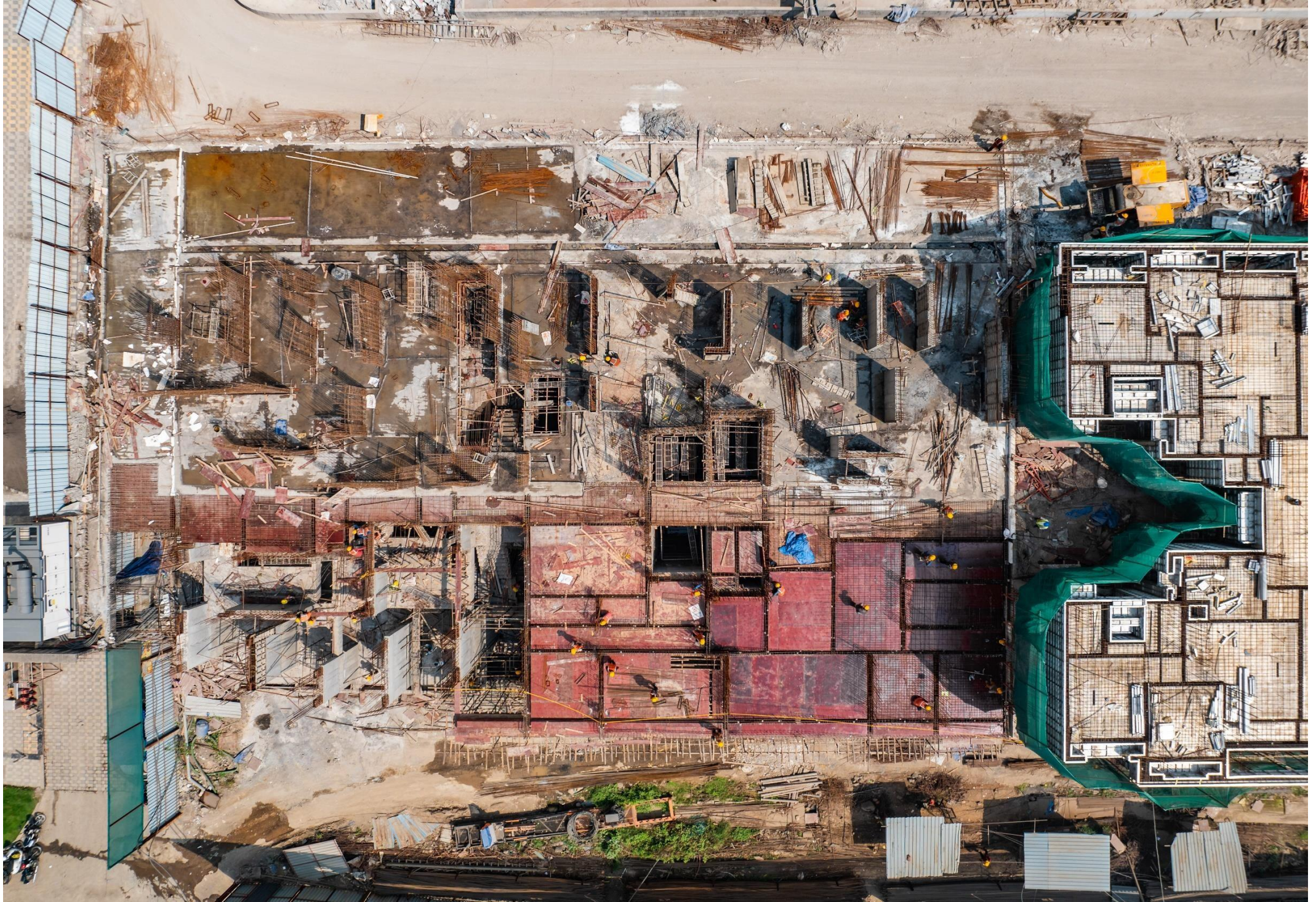
OLIVE A - 1 ST FLOOR LEVEL SLAB WORK IN PROGRESS & OLIVE B - 2 ND FLOOR LEVEL SLAB IN PROGRESS.
