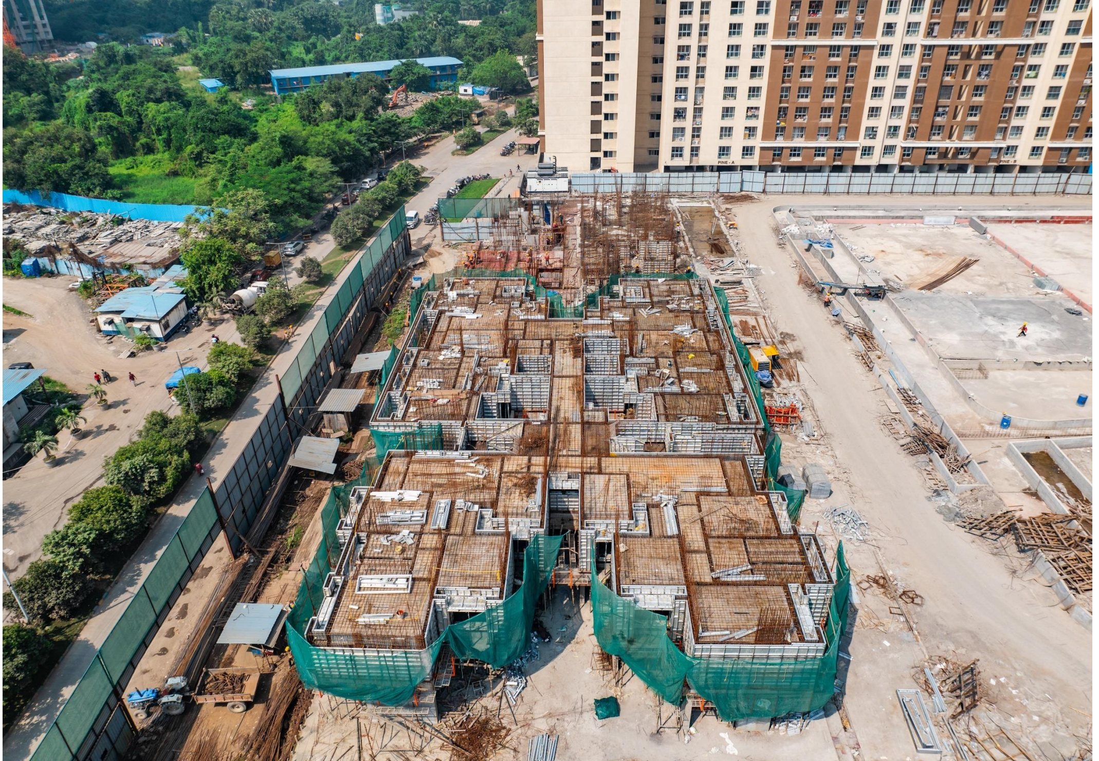
OLIVE A - 1 ST FLOOR LEVEL SLAB WORK IN PROGRESS & OLIVE B - 2 ND FLOOR LEVEL SLAB IN PROGRESS.
