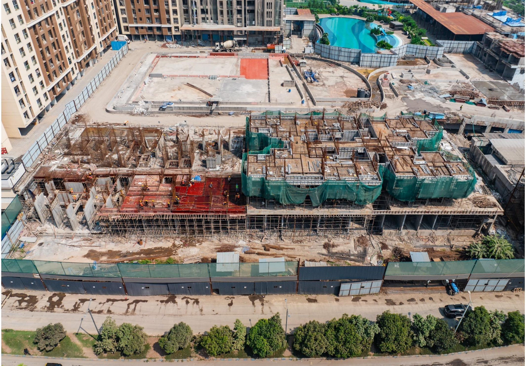
OLIVE A - 1 ST FLOOR LEVEL SLAB WORK IN PROGRESS & OLIVE B - 2 ND FLOOR LEVEL SLAB IN PROGRESS.
