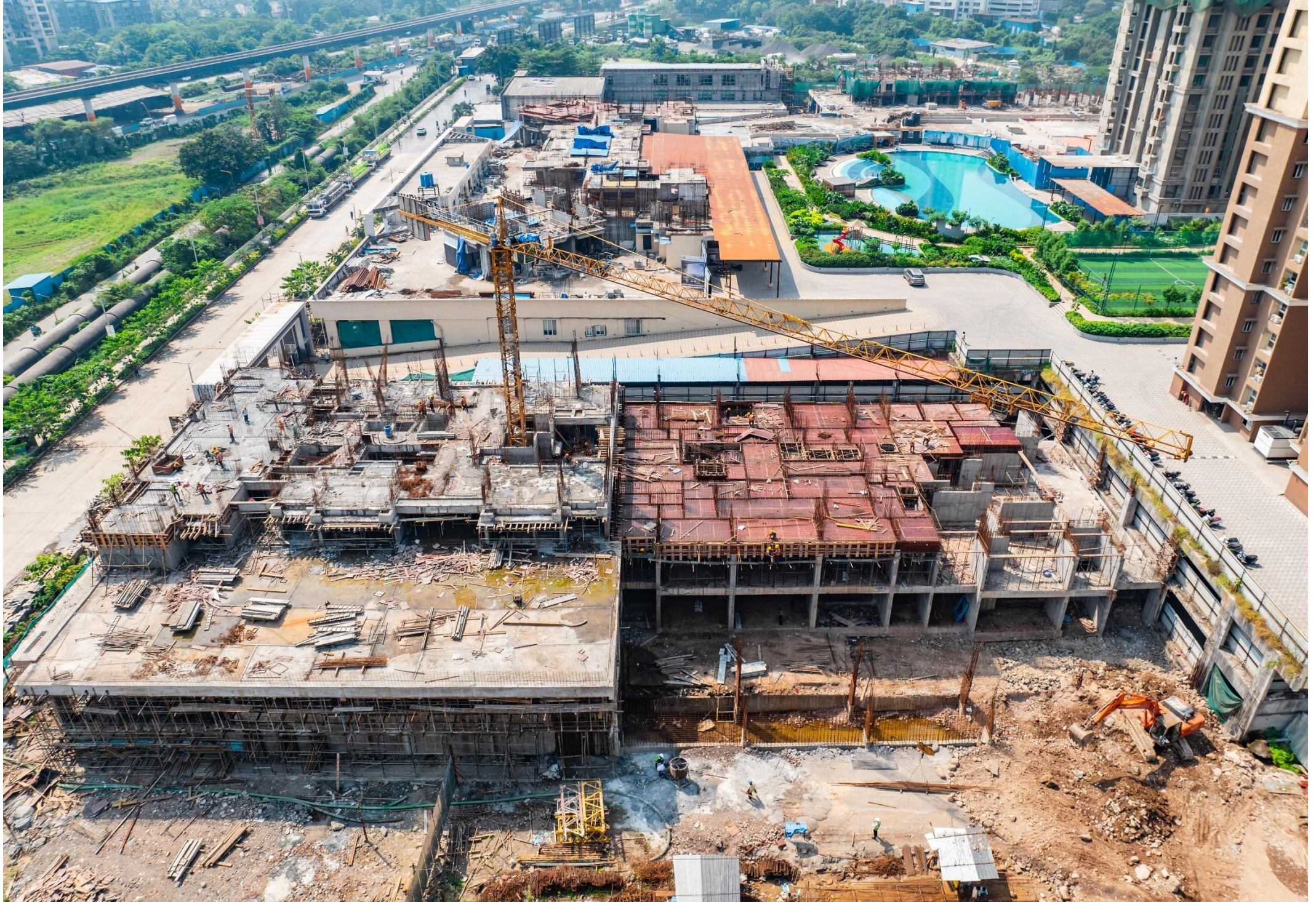
MAPLE A WING - PODIUM FLOOR LEVEL SLAB WORK IN PROGRESS & MAPLE B WING - 1 ST FLOOR LEVEL SLAB WORK COMPLETED
