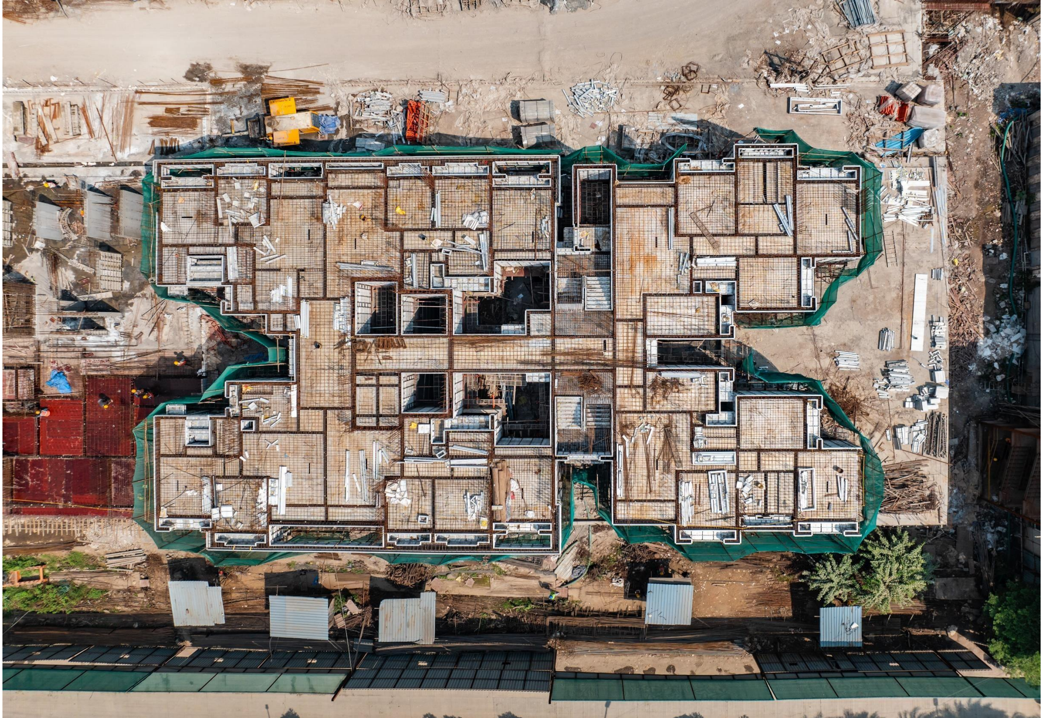
OLIVE A - 1 ST FLOOR LEVEL SLAB WORK IN PROGRESS & OLIVE B - 2 ND FLOOR LEVEL SLAB IN PROGRESS.
