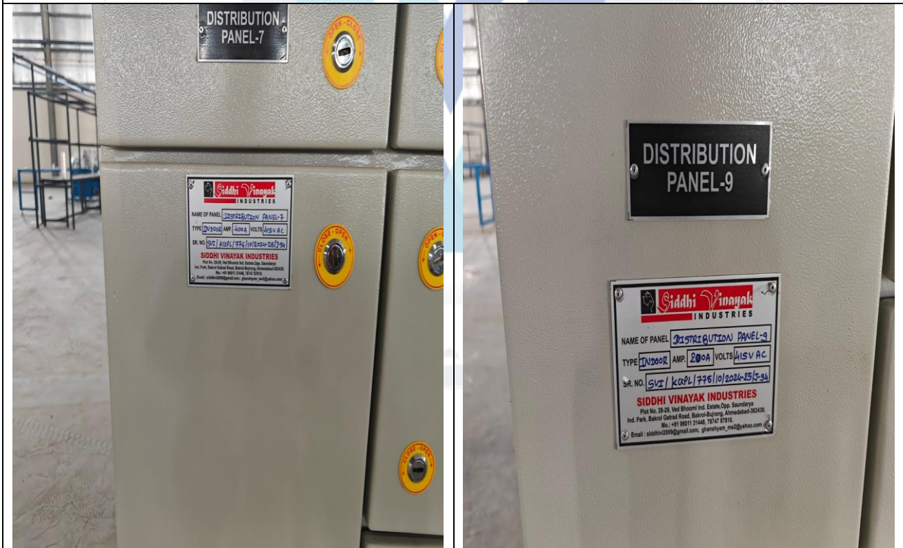
View of Supply of Distribution Panels (DB-1 to DB-14) - Installed
