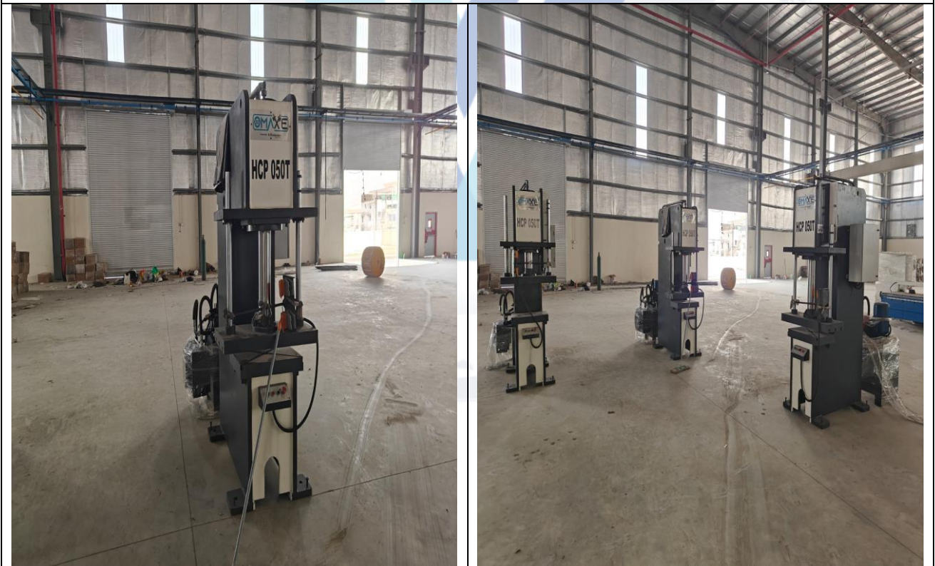
View of Hydraulic C Frame Press - HCP 50T- Kept in Shed
