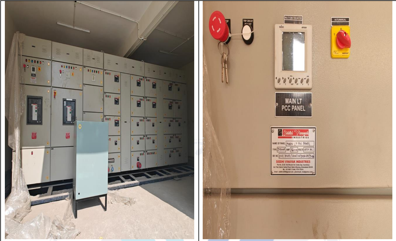
View of Supply of Main Panel, Indent No. 2425-KGPL-IND-100012- Installed
