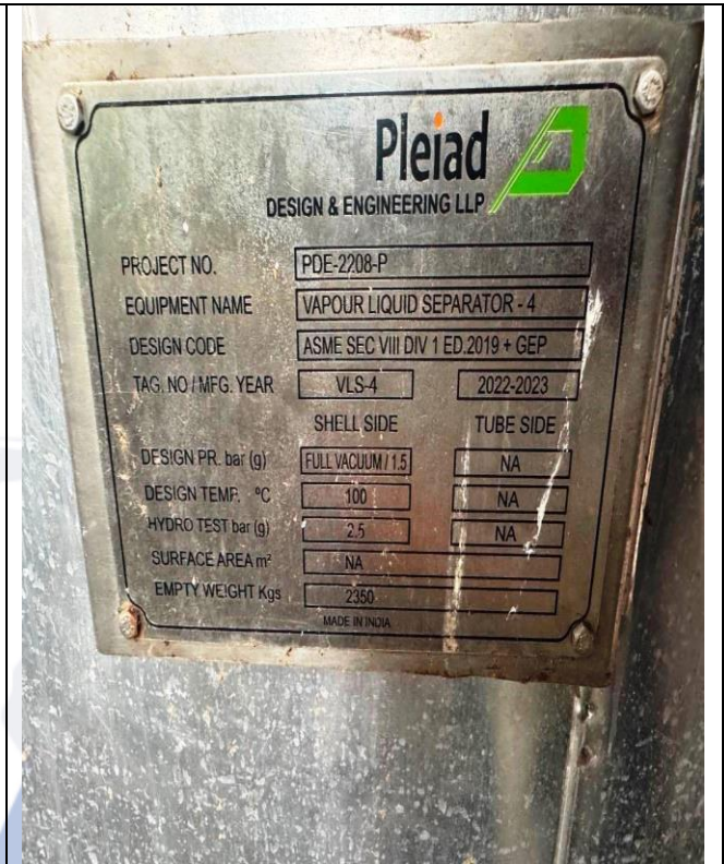
Name Plate of Vapour Liquid Separator-4
