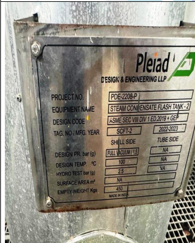
Name Plate of Steam Condensate Flash Tank-2
