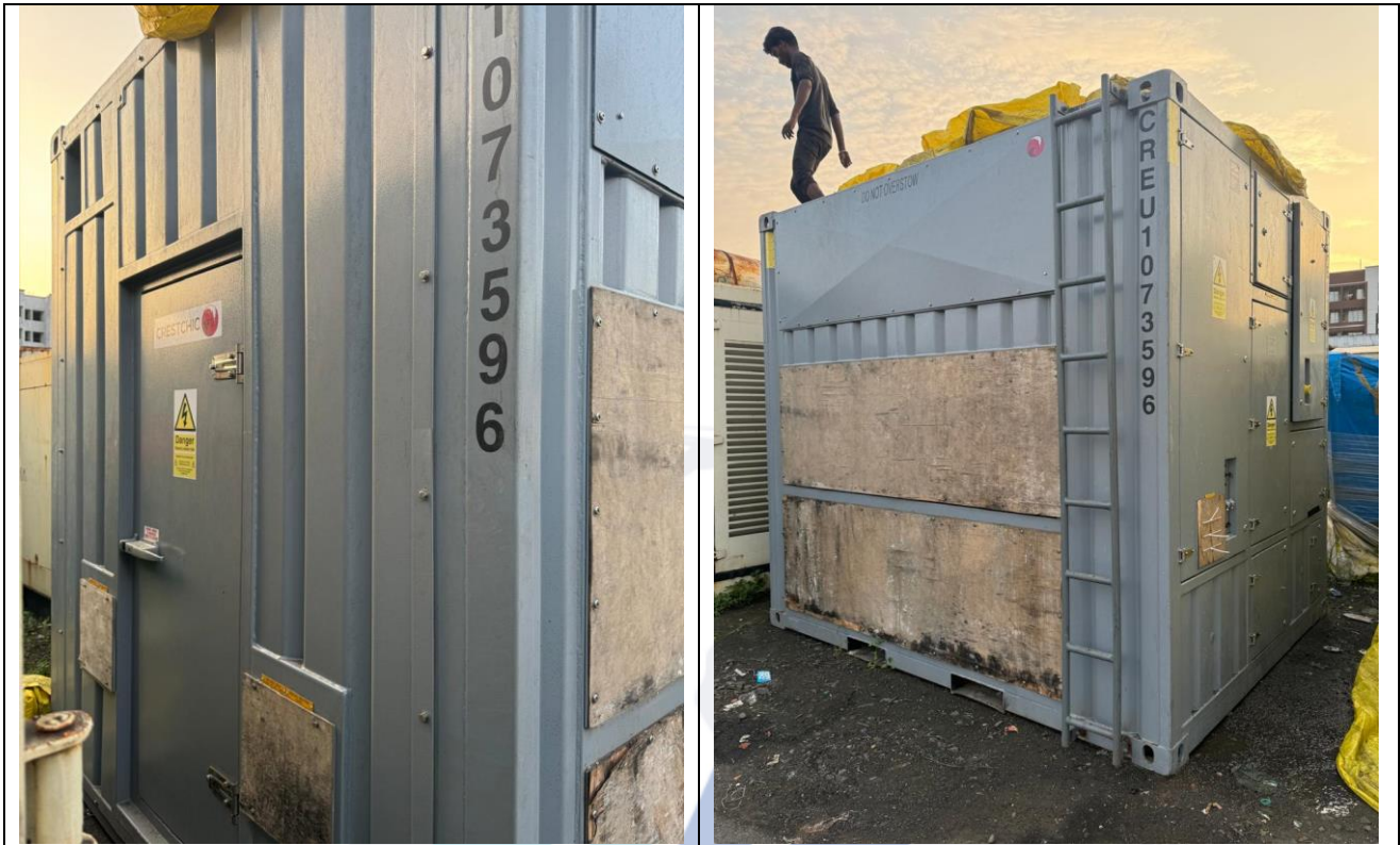
View of 3300 kVA Load Bank, Sr. No. C7359 at Location-3
