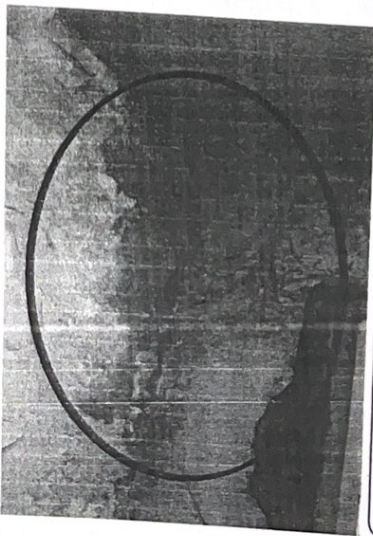
2. B-SEVERE EXTERNAL SEEPAGE IN CEILING IS OBSERVED.
