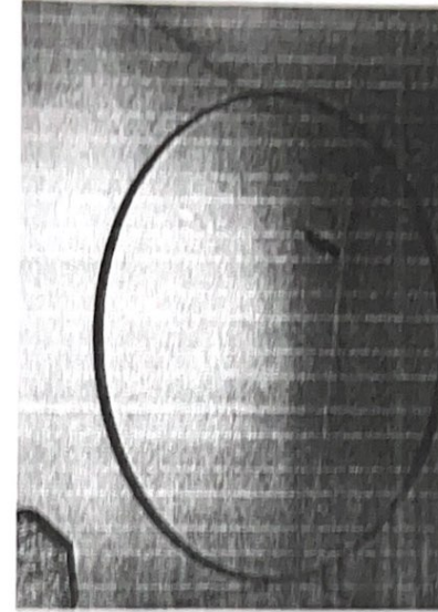
1.A- CEILING SHOWS DELAMINATION EFFECTS.
