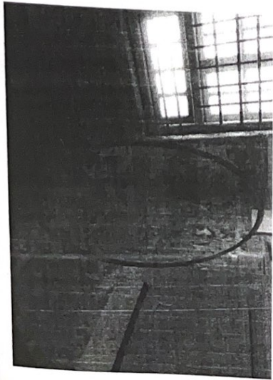
2. B- EXTERNAL SEEPAGE WITH DEEP MASONRY CRACKS IS FILLED WITH CEMENT MORTAR.
