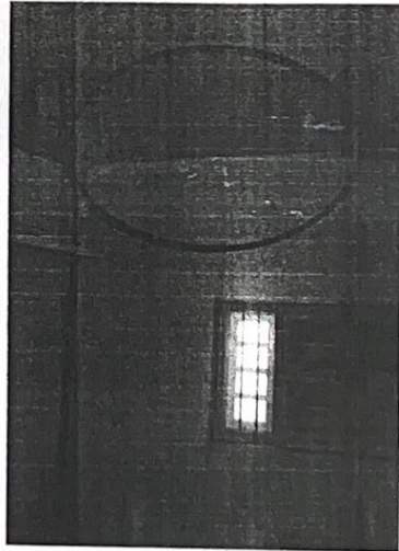
2. B- LOAD BEARING MASONRY WALLS SHOWS EXTERNAL SEEPAGE.
