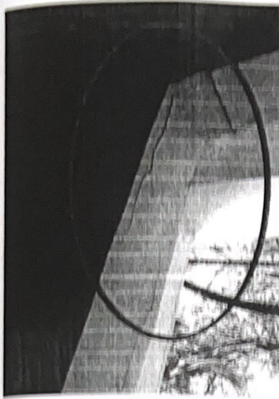
1.A- RC CRACK DEVELOPED IN THE R.C.C. BEAM
