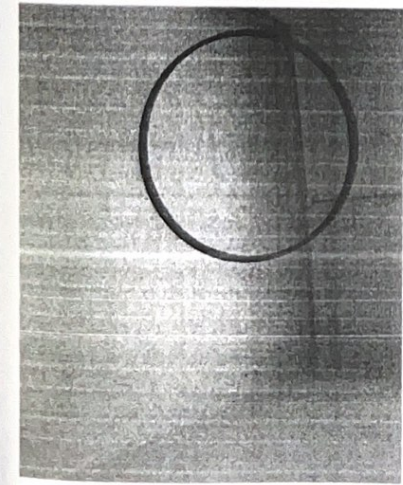
5.B- CEILING SHOWS CRACKS & CRAZING.
