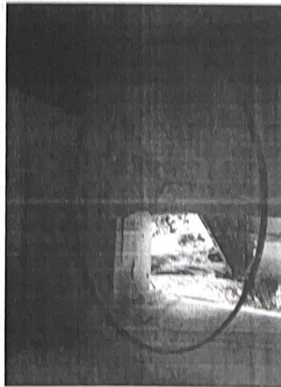
1.A- VERTICAL CRACK IN LOAD BEARING WALL MASONRY IS OBSERVED.
