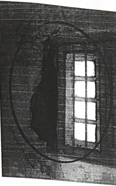
2. B- SEVERE STEEL EXPOSED AT R.C.C BEAM IS OBSERVED.
