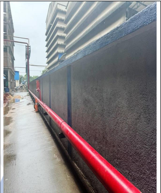
Fire Hydrant System
