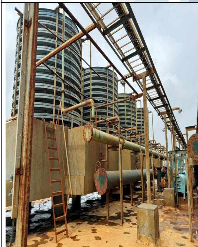
FRP Counter Flow Cooling Tower- 300 TR
