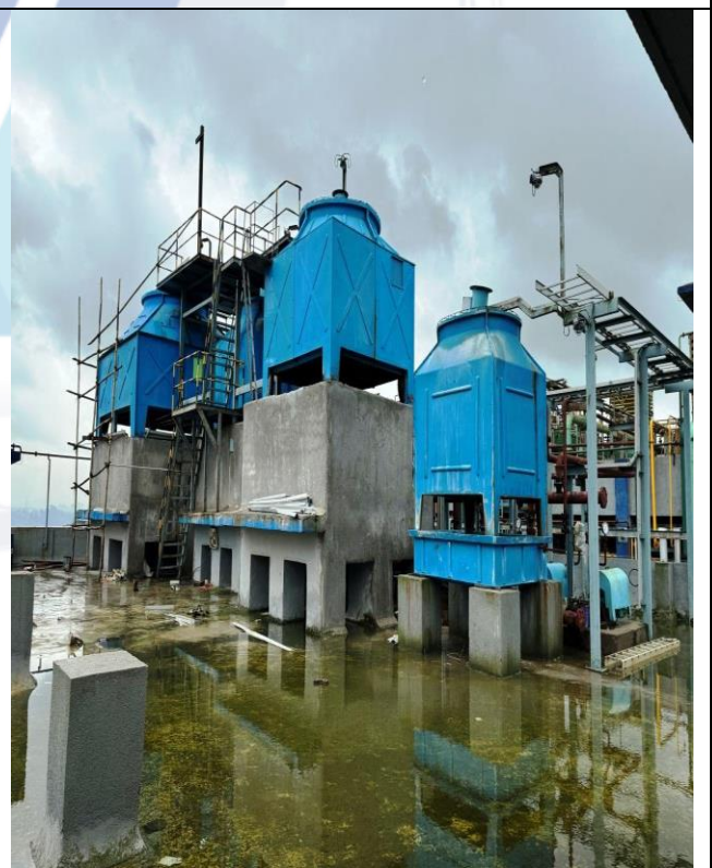
Utility Tower- 650, 300, 225 & 100 TR
