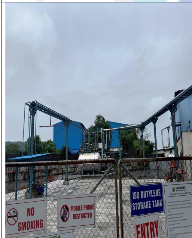
Storage Tank- 19.8 m 3
