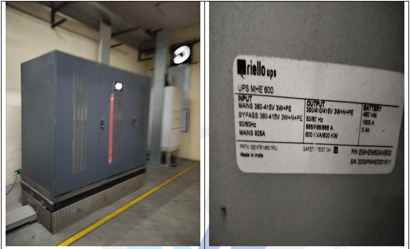
UPS MHE 600KVA, Sr. No. 2008PMHE0001611 at Location-4
