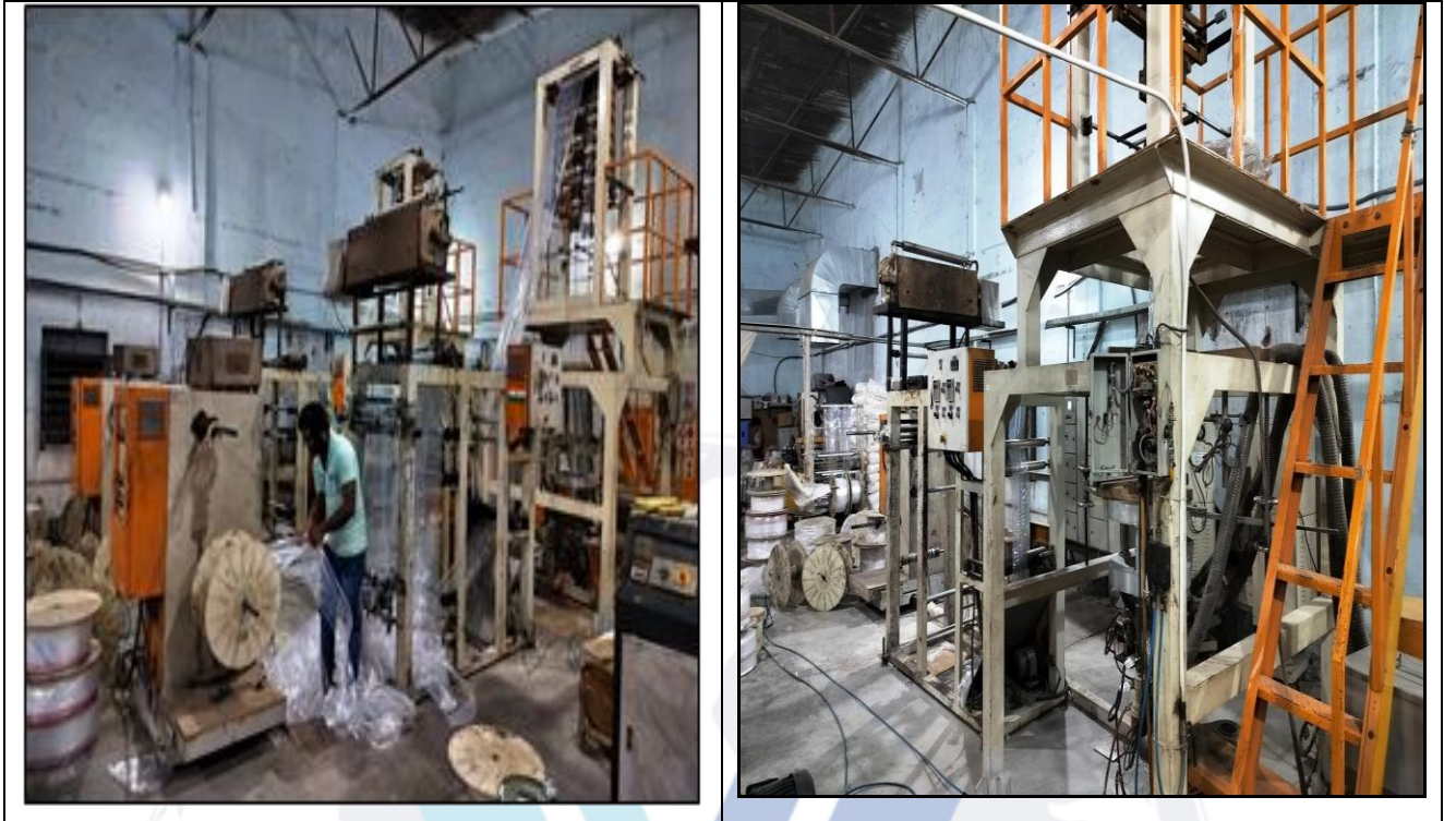
LPE High Speed Zipper Film Inflation machines 2 sets Model AEZ-45, Sr. No. 20130714 at Location-1
