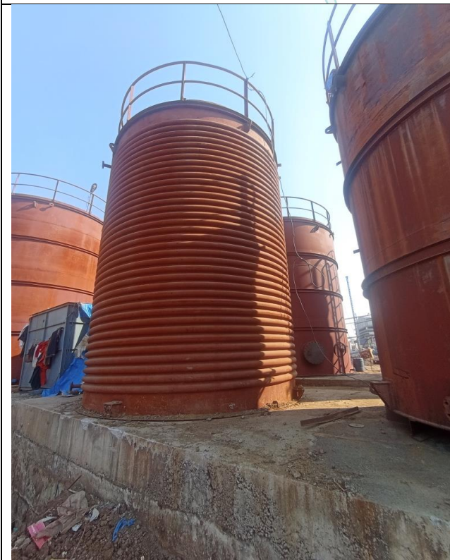
MS Storage Tank
