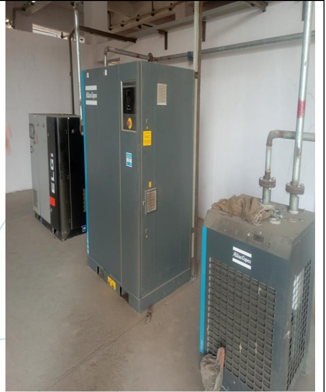
Air Compressor & Dryer
