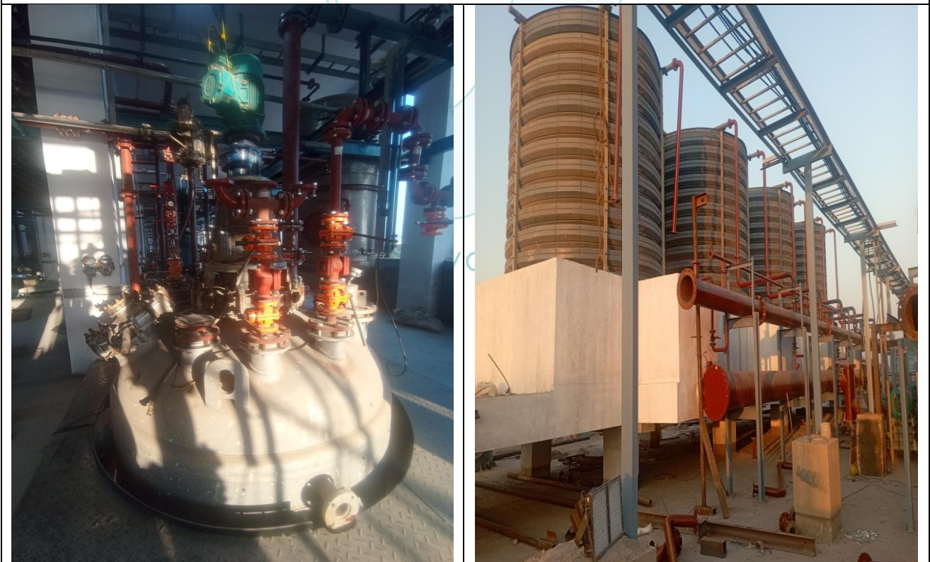
MS Glass lined Jacketed Reactor
