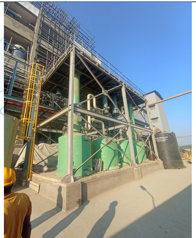
Utility Cooling Tower
