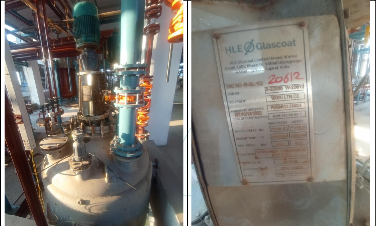
MS Glass lined Jacketed Reactor
