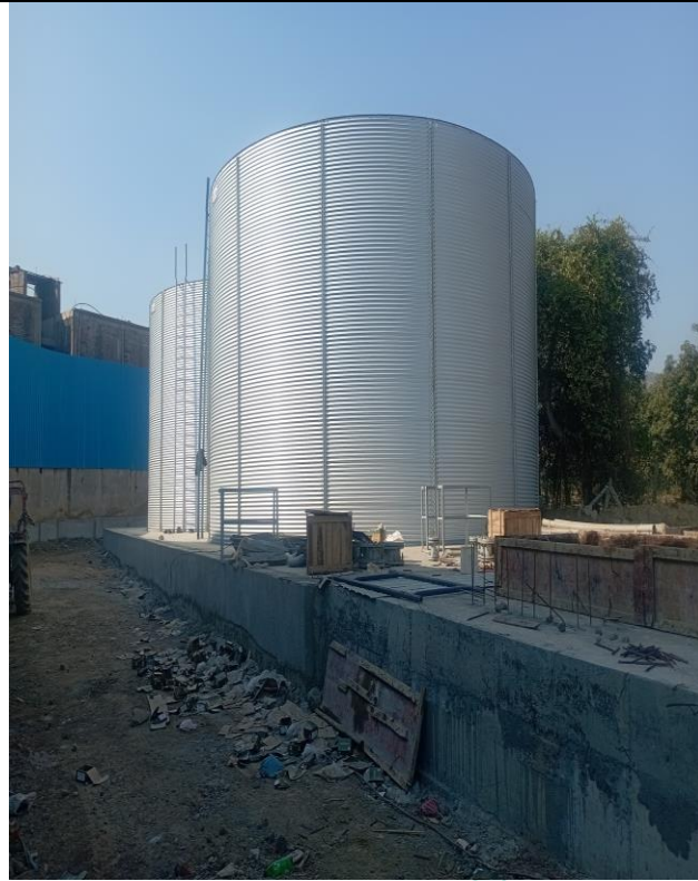
Fire Water Tank
