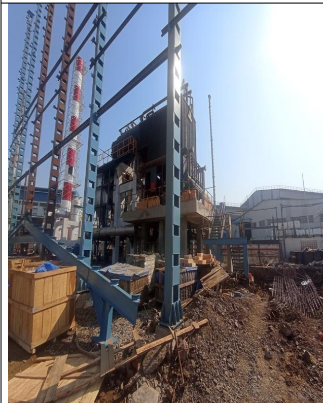
View of Boiler & ESP
