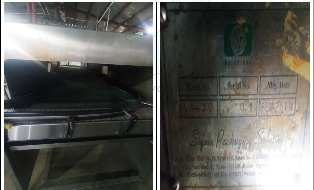
View of Cooling tunnel for Juice Filling Plant, Sr. No. 1 and SS Chain Conveyor
