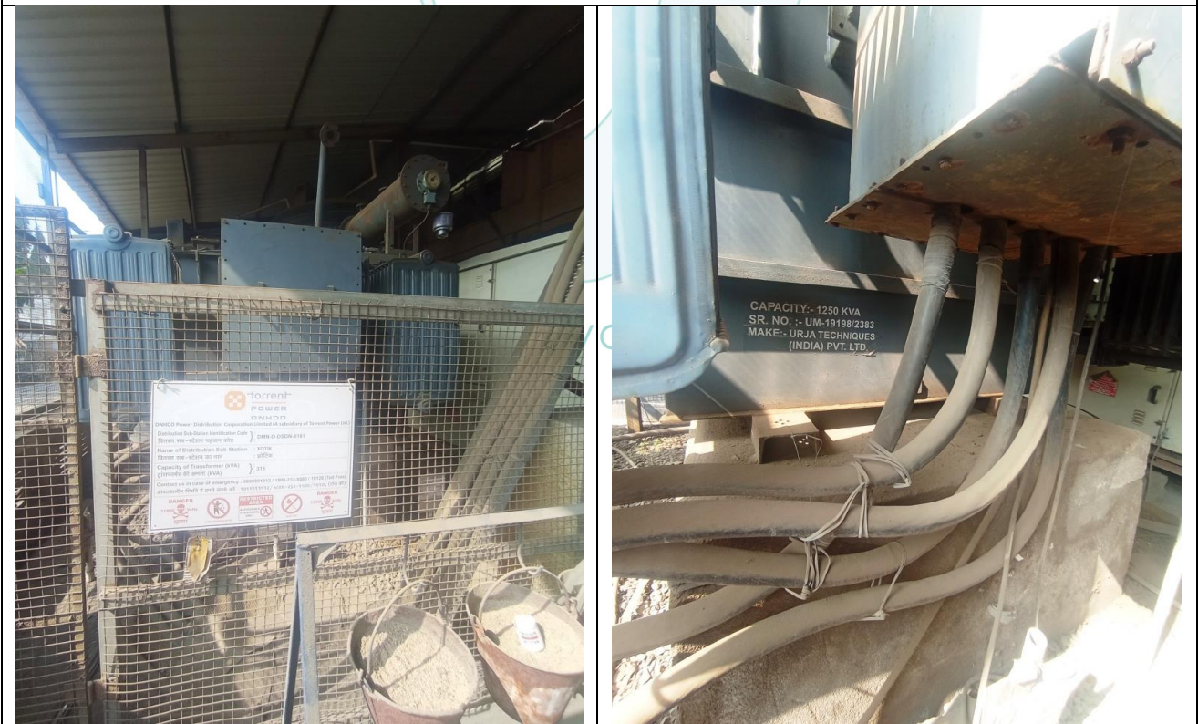
View of Distribution Transformer 1250 KVA, 11/0.433kv, Sr. No. UM-19198/2383
