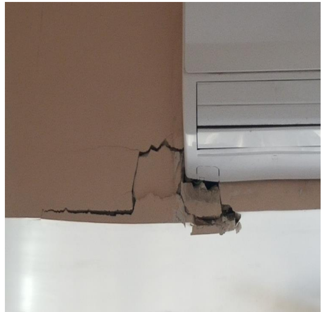
Flat No. 401A: cracks on beam at bedroom-2
