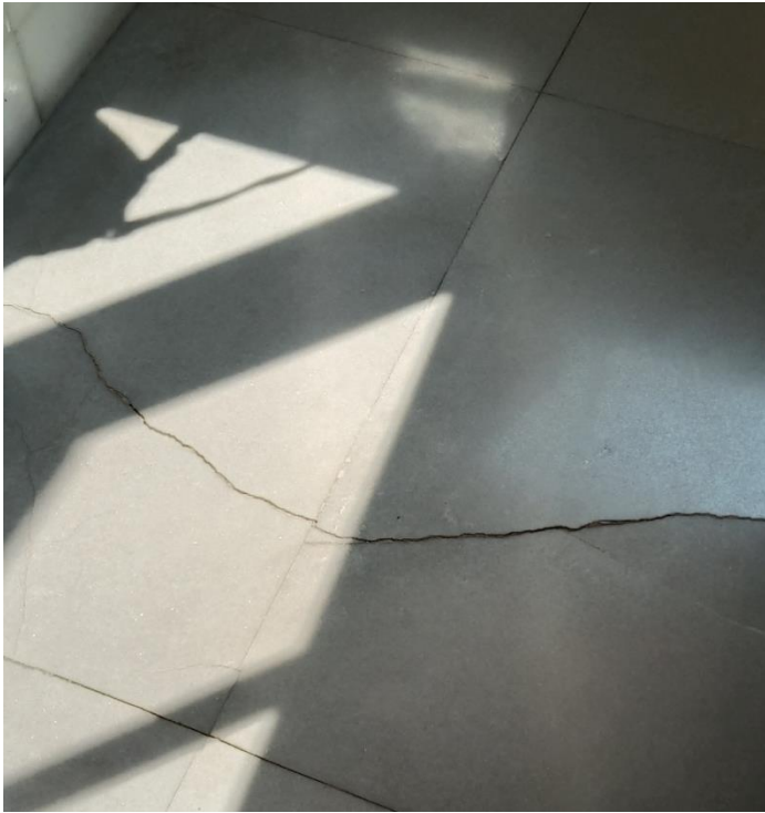
Flat No.509: cracks on floor tiles/stone
