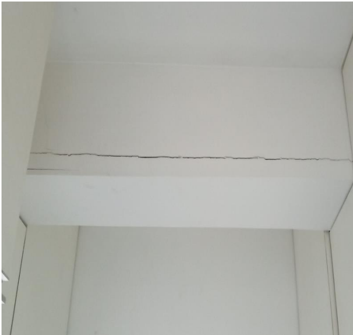
Flat No. 107: Cracks on beam at bedroom
