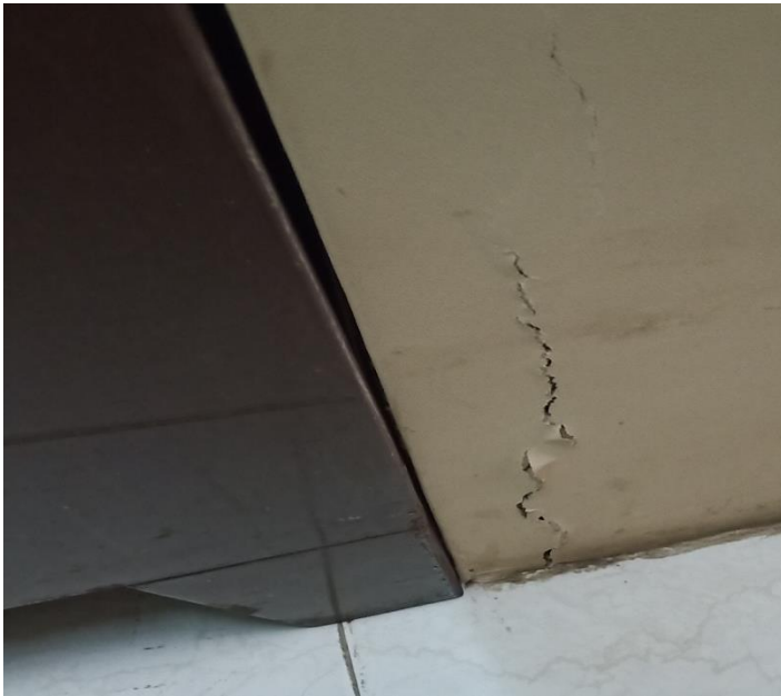
Flat No. 206: Cracks on column at bedroom
