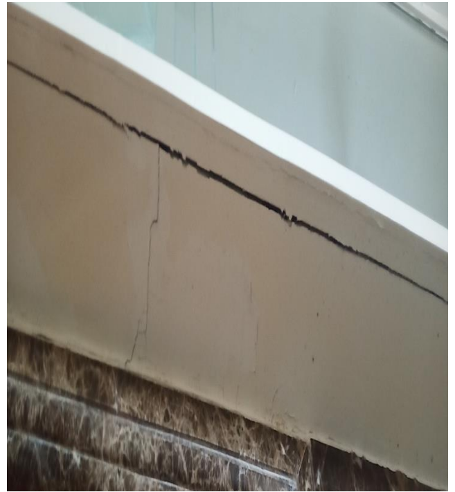
Flat No.502: cracks on beam at bedroom-6
