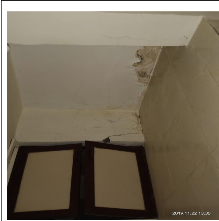
Flat No. 308: leakage marks on ceiling
