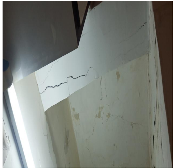
Flat No.508: cracks on beam bottom
