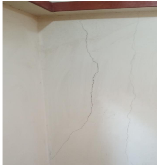
Flat No. 110: Cracks on on column at bedroom
