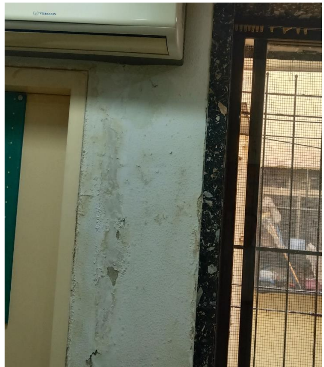
Flat No.408: leakage marks on chowk side wall
