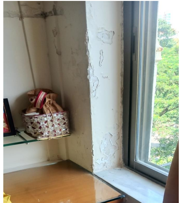
Flat No.510: leakage marks on external wall
