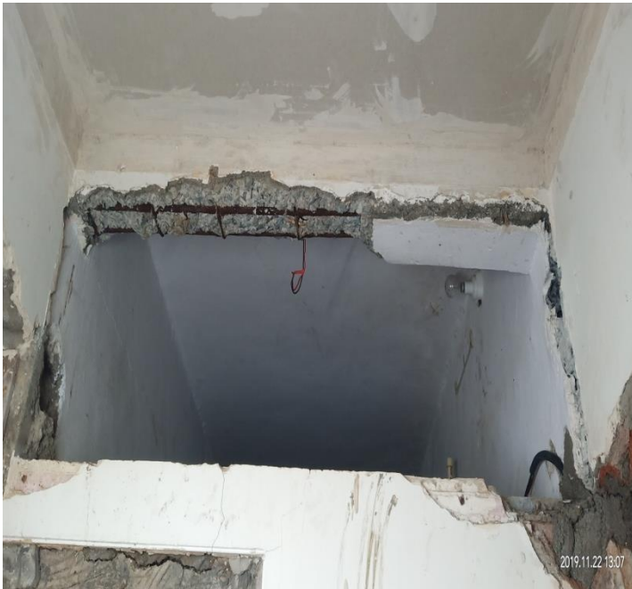
Flat No. 411: corroderd reinforcement at bath
