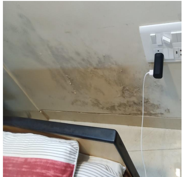
Flat No. 105: Leakages marks on wall at bedroom-2
