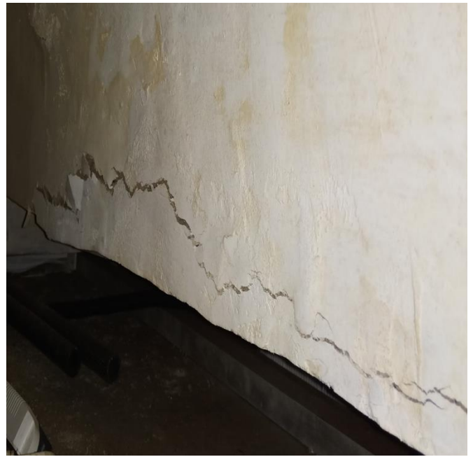
Shop No. 3: Wide cracks on RRC Beam
