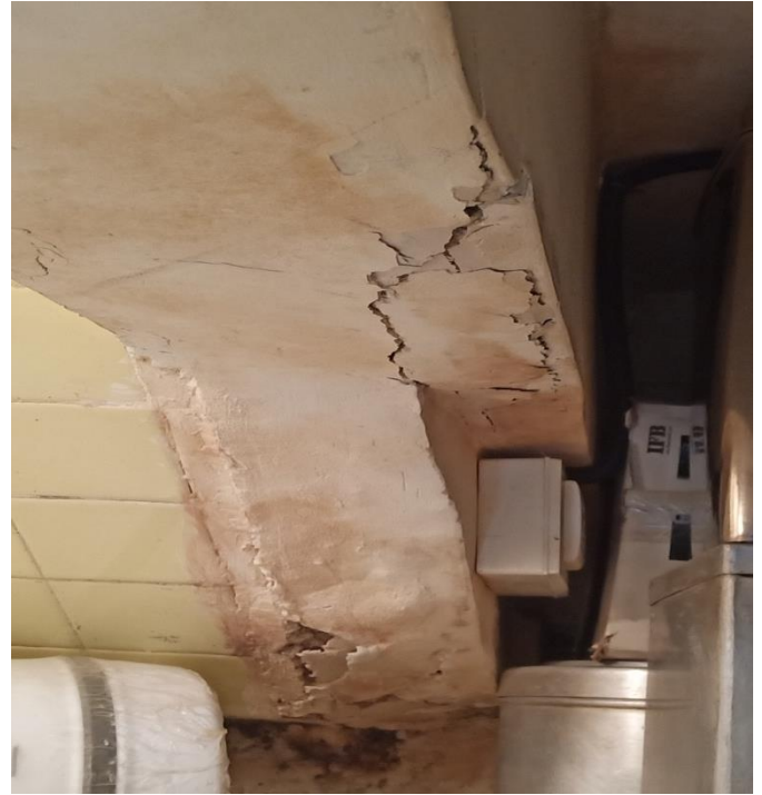
Flat No.408: cracks on beam
