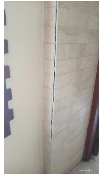
Flat No. 104: Tiles cracks on column
