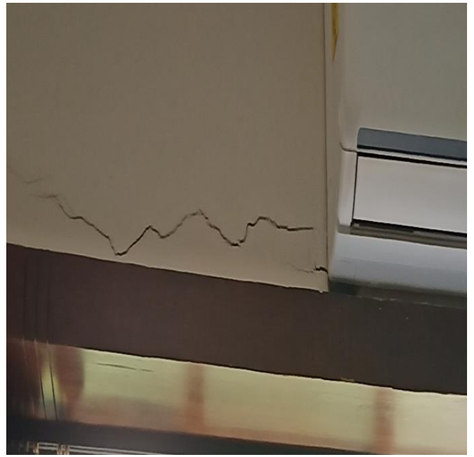
Flat No. 311: cracks on column at bedroom -2
