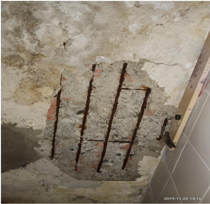
Flat No. 401A: exposed of reinforcement on bedroom ceiling
