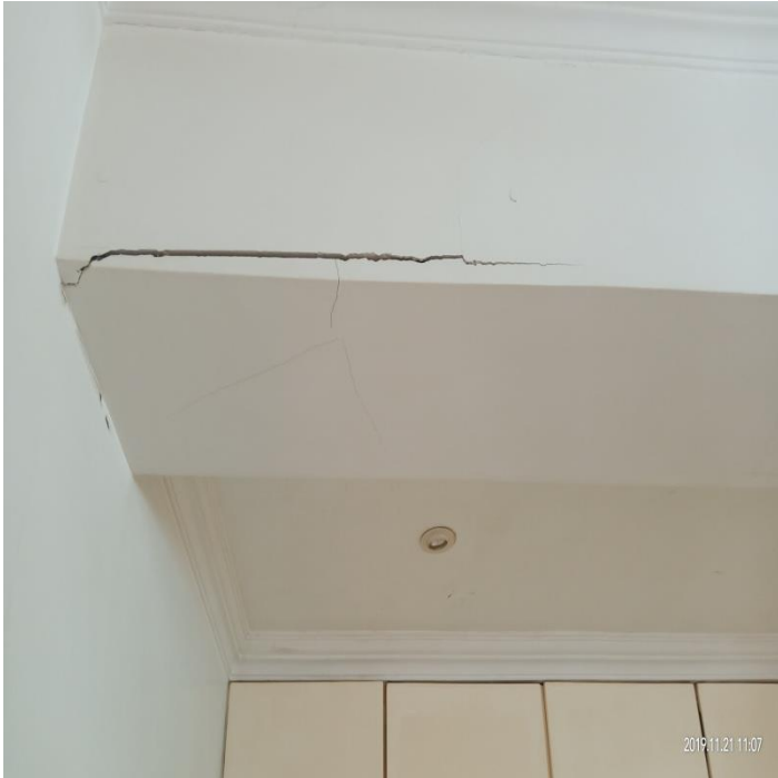
Flat No. 503: cracks on beam bottom at bedroom-3
