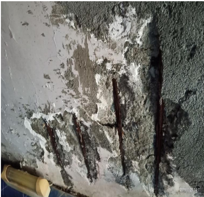
Flat No. 205: exposed of reinforcement on loft ceiling.
