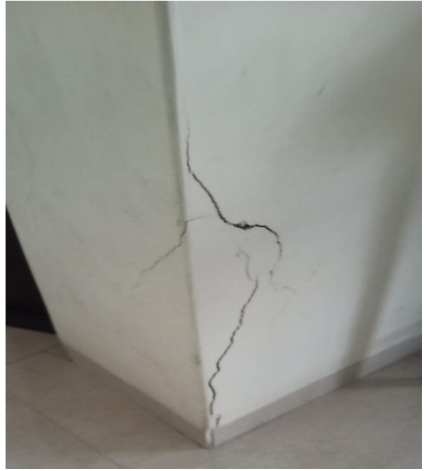
Flat No. 205: Wide cracks on column at livingroom
