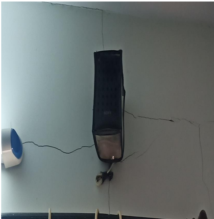
Flat No.505: cracks on beam at bedroom-1
