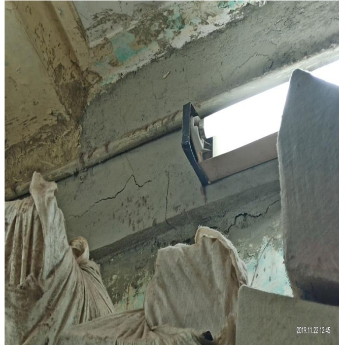
Flat No. 307: Cracks on beam at kitchen
