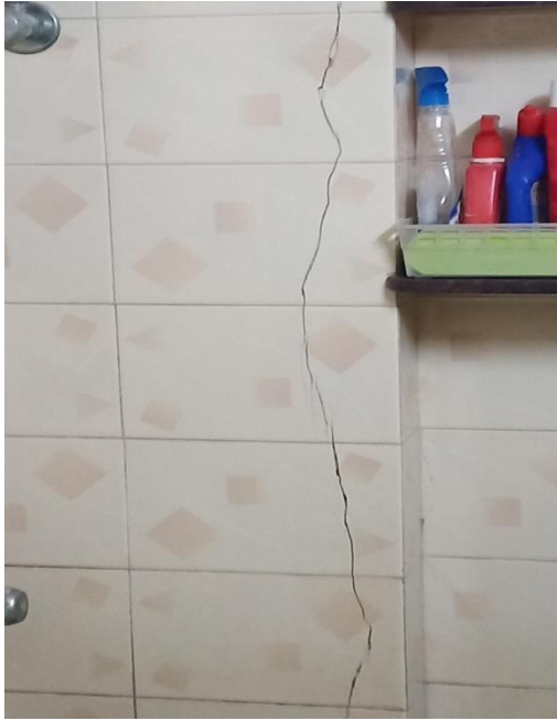
Flat No. 306: Tiles cracks on column at bathroom
