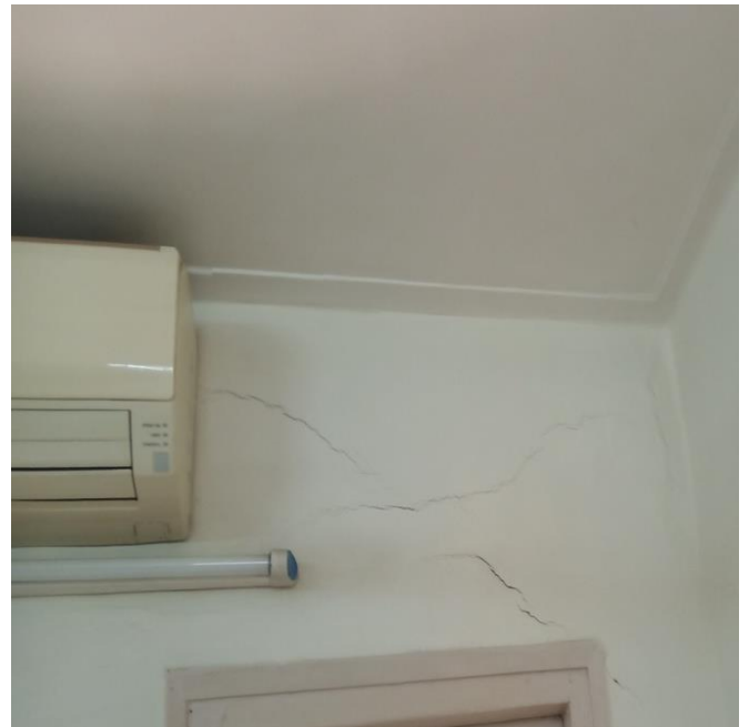
Flat No.508: cracks on beam bottom
