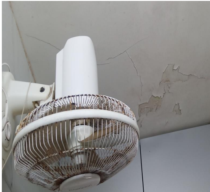
Flat No. 104A: Cracks on ceiling
