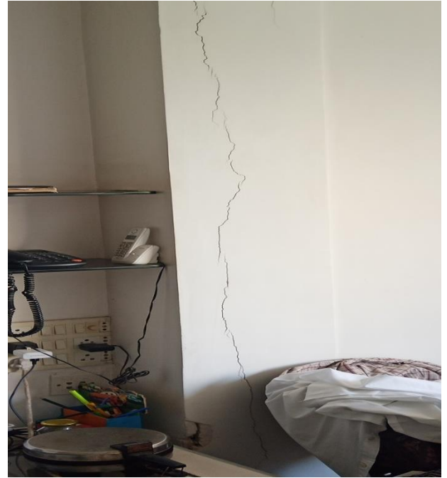
Flat No. 401A: vertical cracks on column at living room
