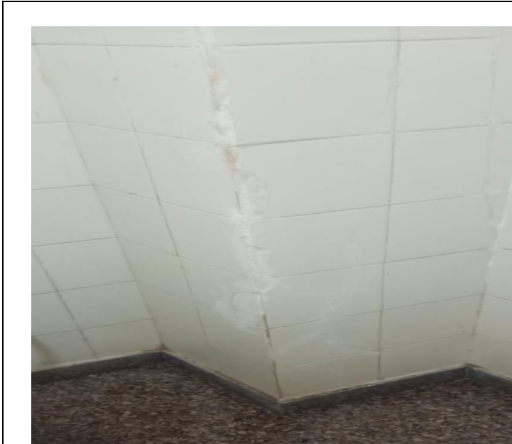
Flat No. 501: Tiles cracks on bathroom column
