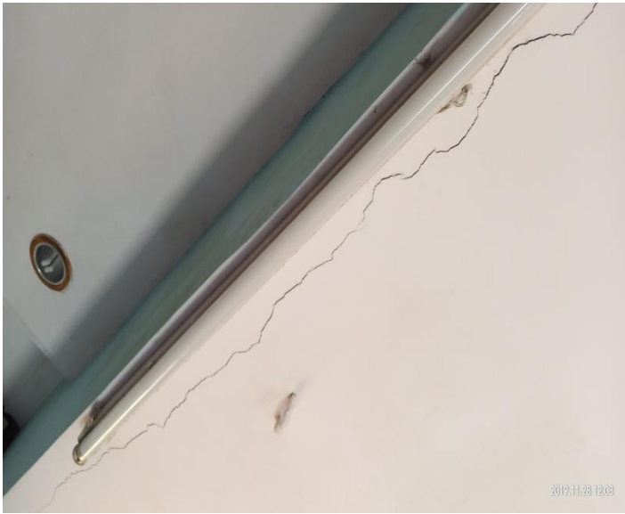
Flat No.506: cracks on beam bottom
