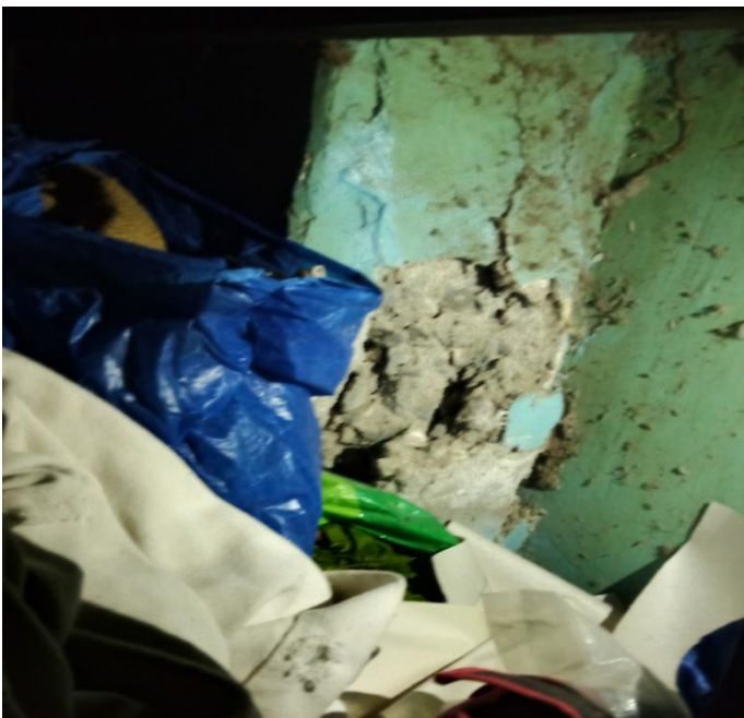
Shop-4: bulging of concrete on ceiling, column and beam
