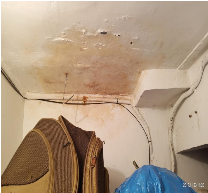
Shop No. 2: Leakage marks on ceiling
