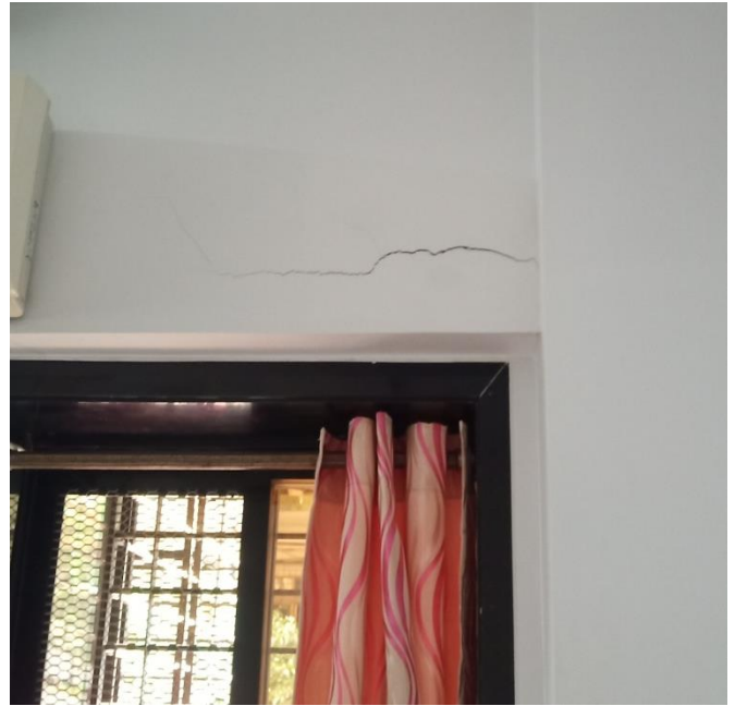
Flat No. 107: Cracks on beam at bedroom
