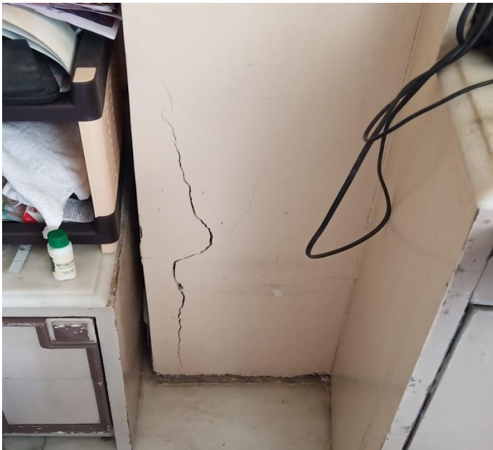
Flat No. 401A: wide cracks on column at bedroom-2
