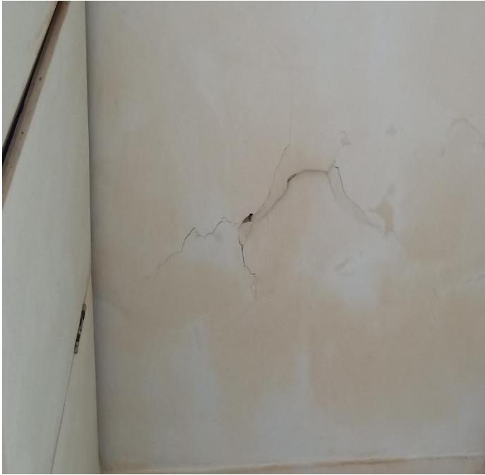
Flat No. 401A: bulging of concrete on ceiling
