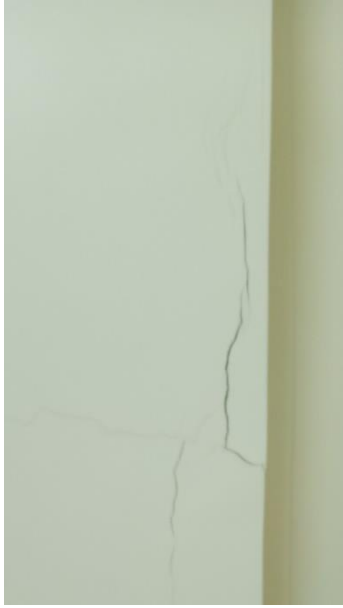
Flat No. 207: cracks on column
