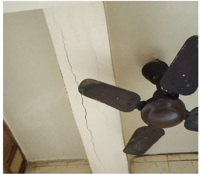
Flat No.506: cracks on beam bottom
