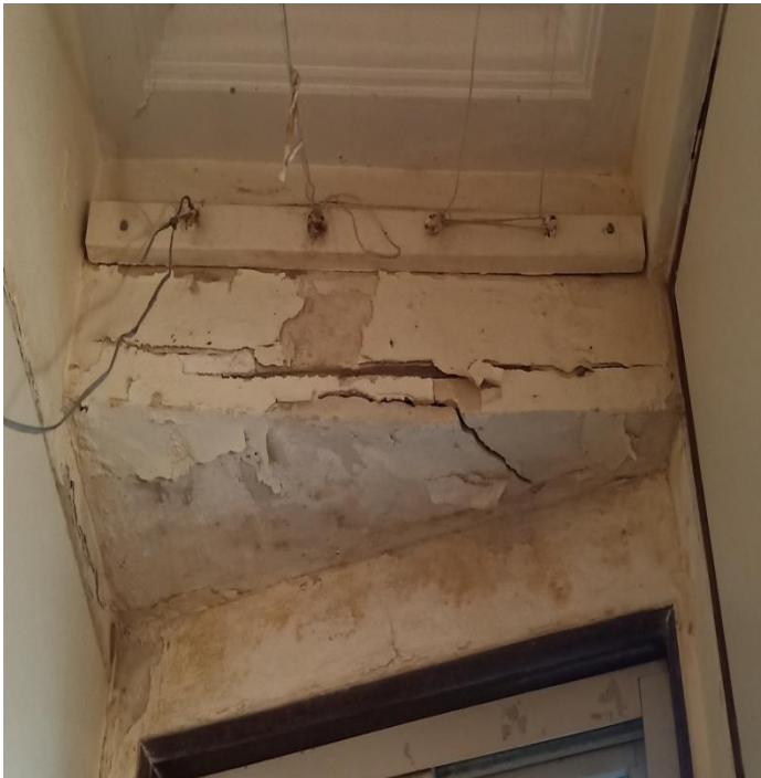
Flat No. 409: cracks on beam
