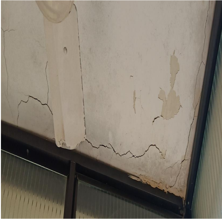
Flat No.408: cracks on ceiling
