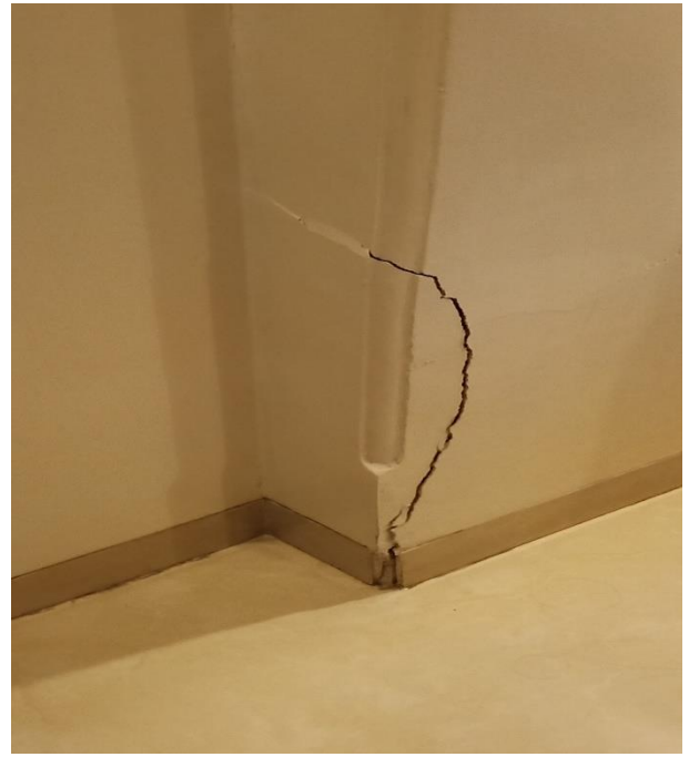
Flat No. 403: Cracks on column at living room
