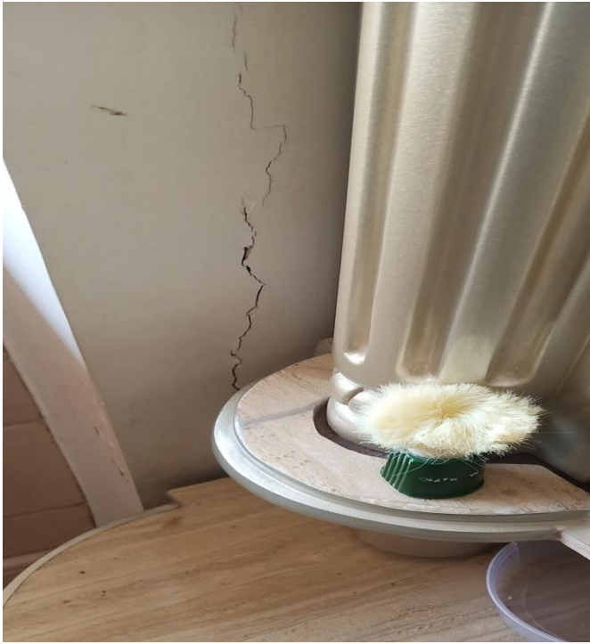
Flat No.503: Cracks on column at bedroom-2
