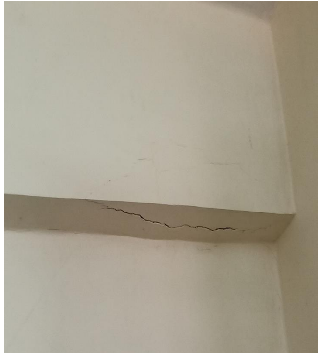
Flat No. 108: Cracks on beam at living room
