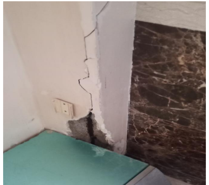
Flat No.502: wide cracks on column at bedroom-1
