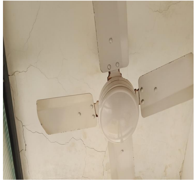
Flat No.408: cracks on ceiling
