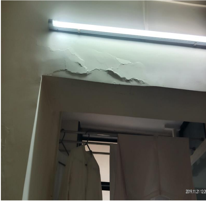
Flat No. 105: Cracks on beam at kitchen
