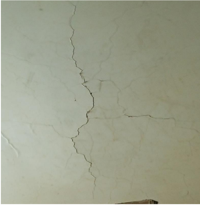
Flat No. 307: cracks on ceiling at bedroom
