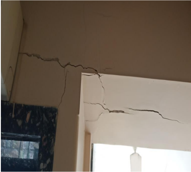
Flat No.408: cracks on beam at bedroom-2
