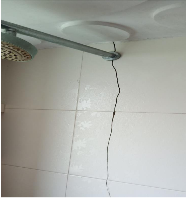
Flat No. 311: Tiles cracks on column at bathroom
