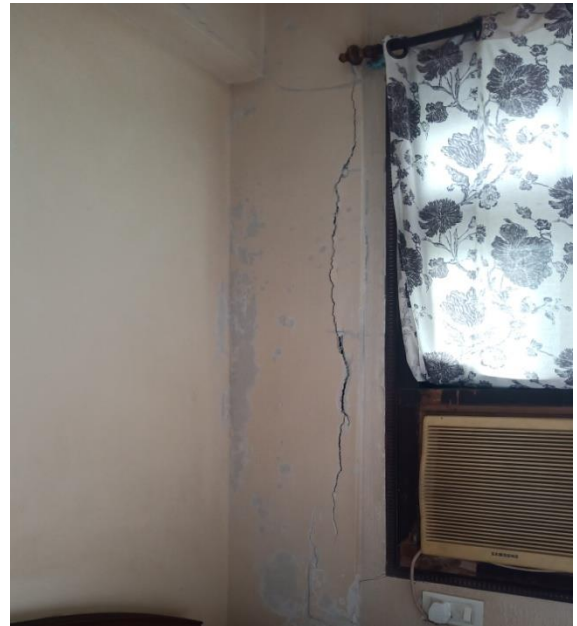
Flat No. 205: Wide cracks on column at bedroom -3
