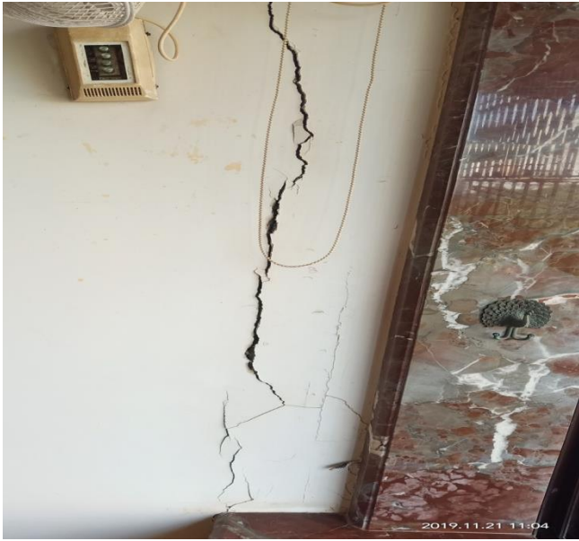
Flat No.503: vertical cracks on living room column
