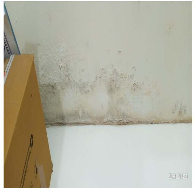
Flat No. 204: Leakage marks on partition wall at Children room
