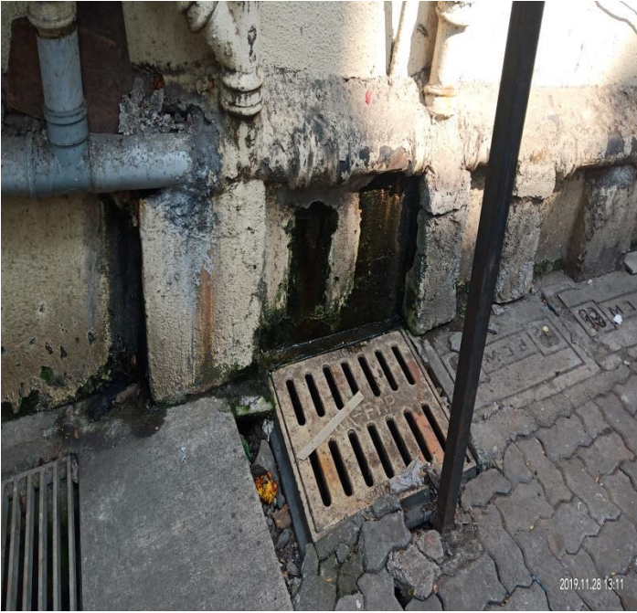
Leakage on Plumbing pipes
