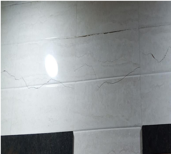
Flat No. 304: Tiles cracks on beam at kitchen
