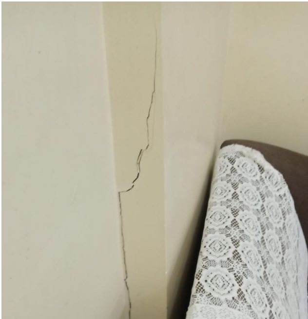
Flat No. 110: Cracks on on column at livingroom
