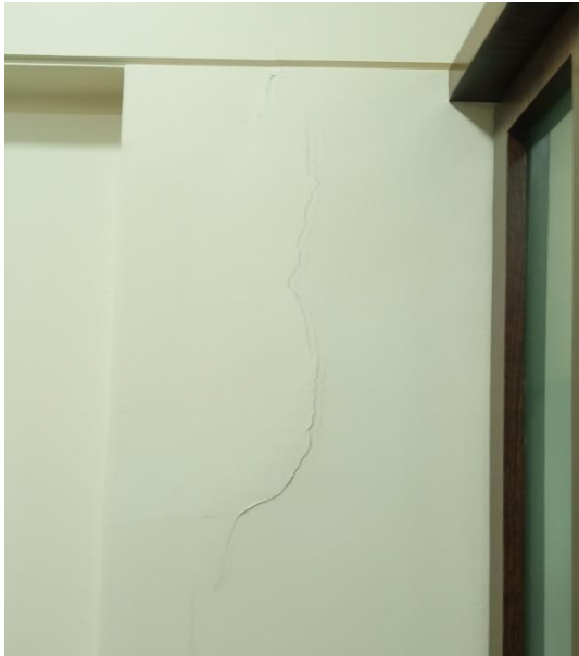
Flat No. 111: cracks on column
