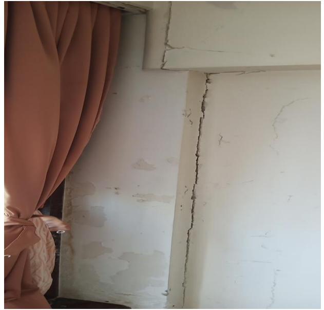
Flat No.503: Cracks on living room column
