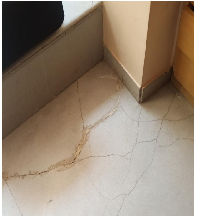
Flat No.509: cracks on floor tiles/stone
