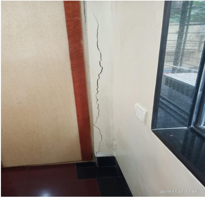
Flat No. 110: Cracks on column at bedroom
