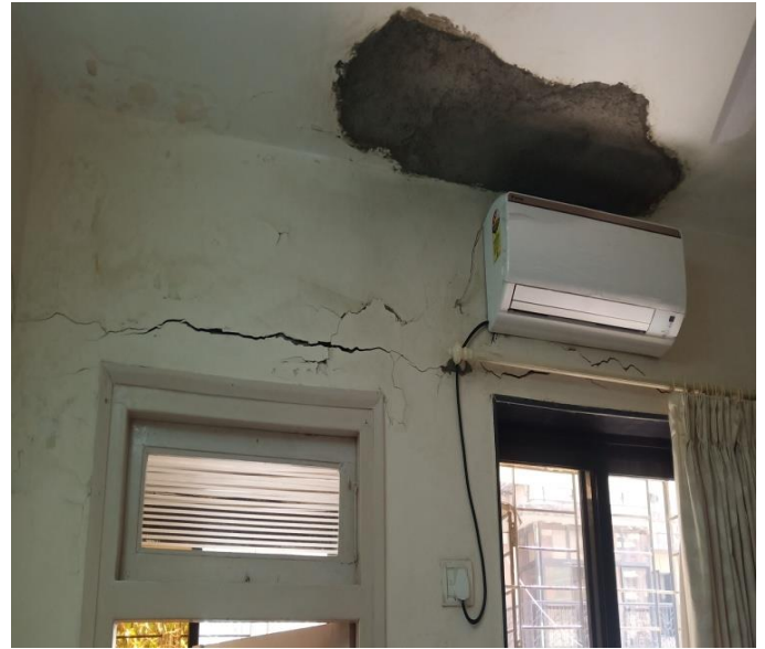
Flat No.508: cracks on beam bottom
