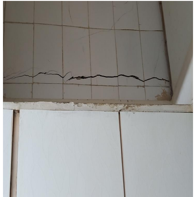
Flat No. 401A: Tiles cracks on beam at kitchen
