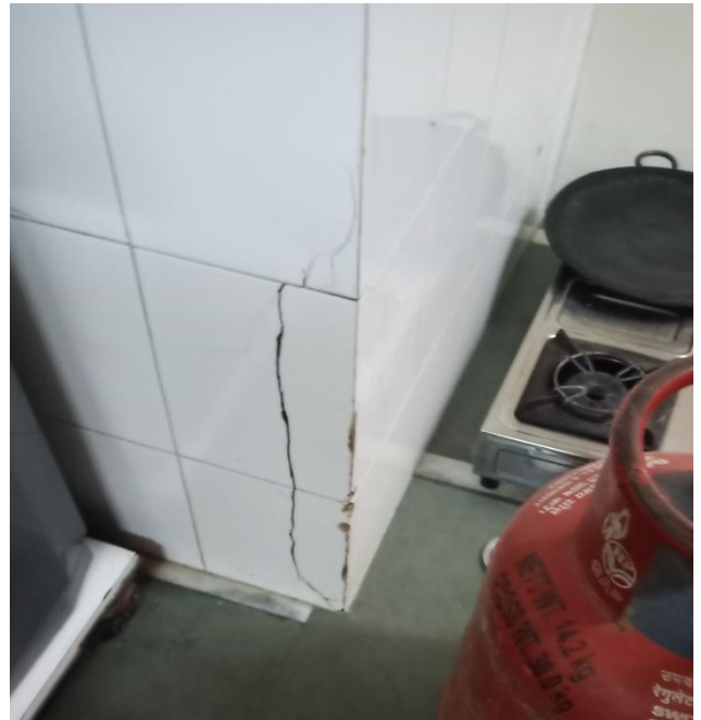
Flat No. 106: Tiles Cracks on column at room
