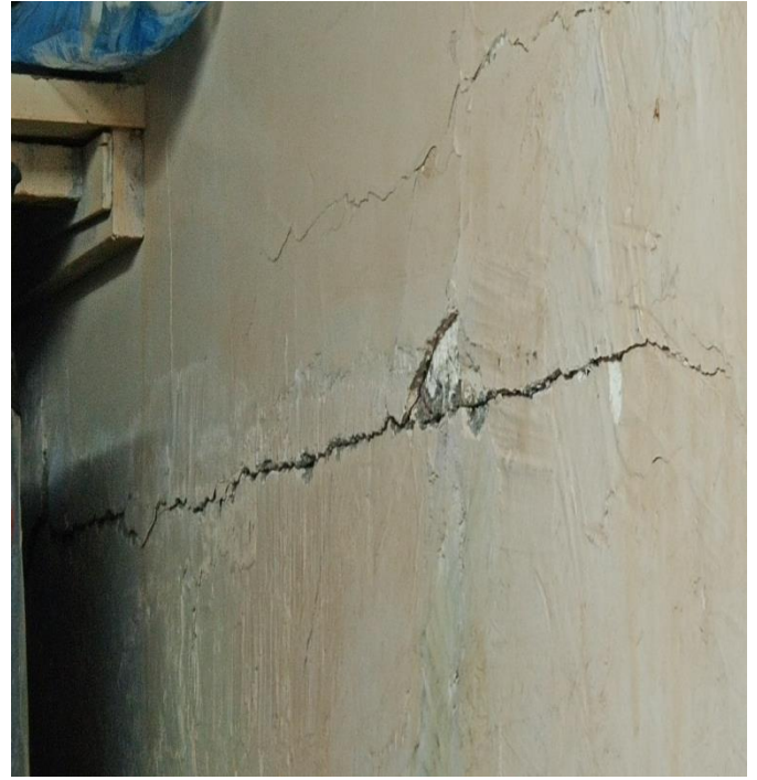
Flat No. 401: Cracks on beam at passage
