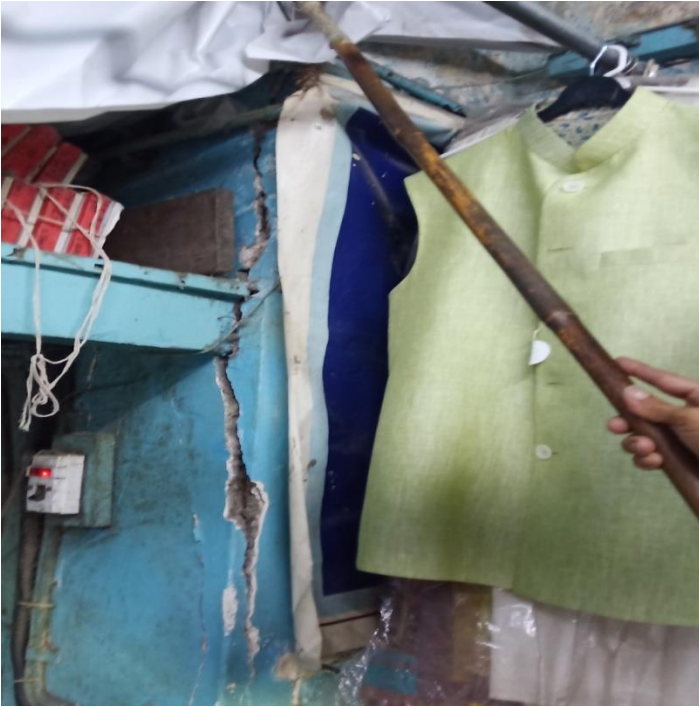
Shop-4: wide cracks on column and bulging of concrete
