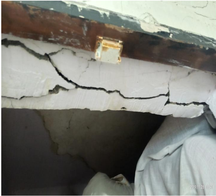
Flat No.508: cracks on beam bottom
