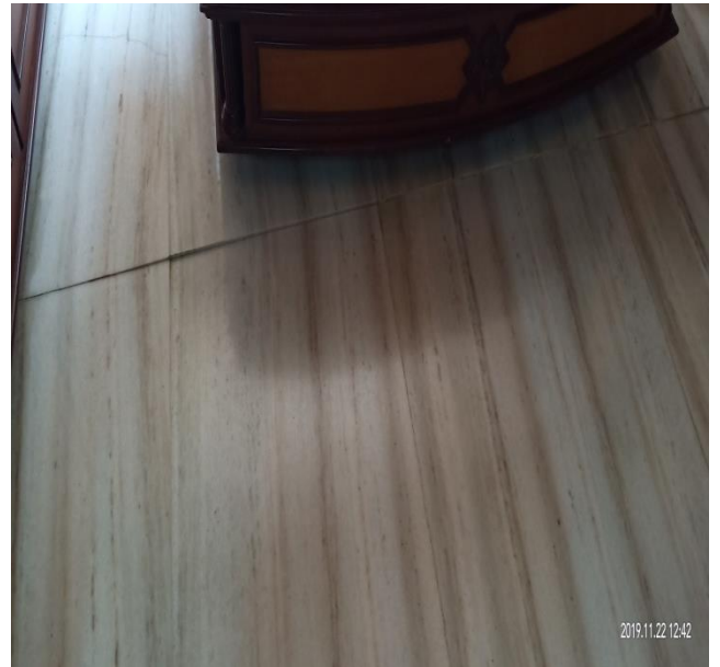
Flat No. 306: Raised on flooring at bedroom
