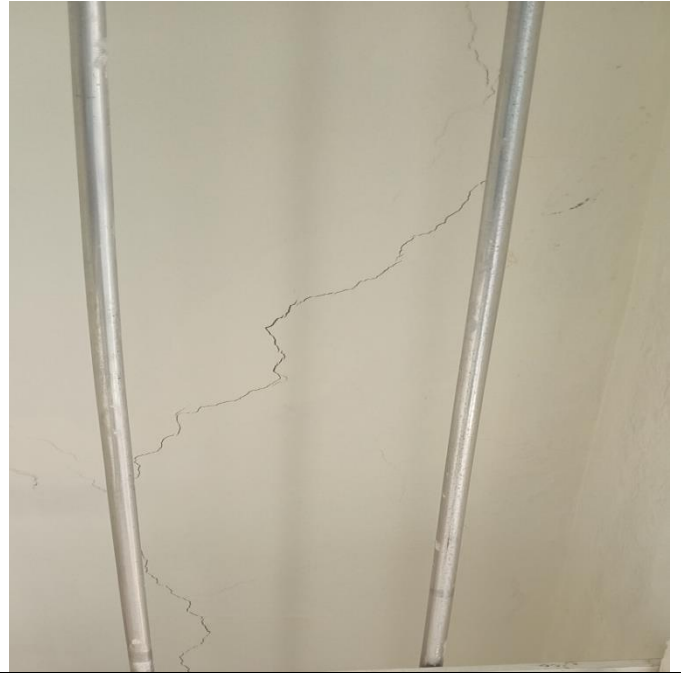
Flat No. 303: Cracks on balcony ceiling at bedroom-2
