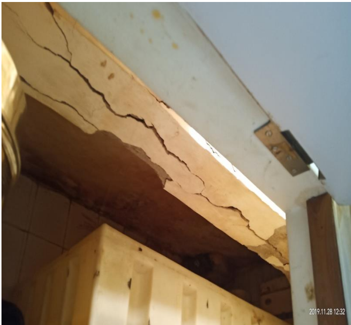
Flat No.408: cracks on beam
