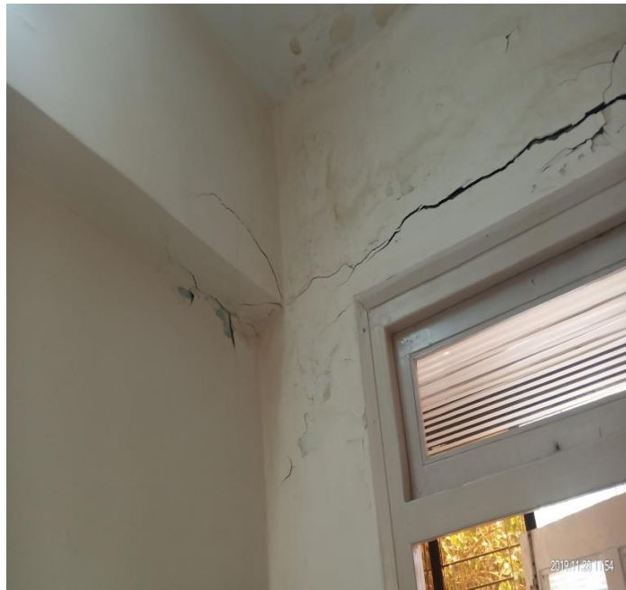
Flat No.508: cracks on beam bottom
