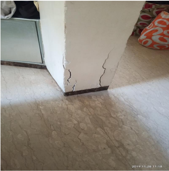
Flat No.502: wide cracks on column at bedroom-1
