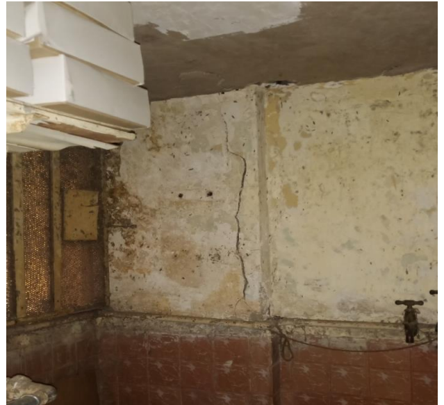
Flat No. 307: Cracks on column at bathroom
