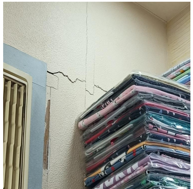
Shop-16: cracks on beam
