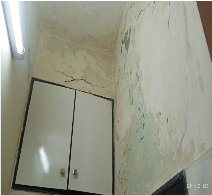
Flat No.508: cracks on beam bottom
