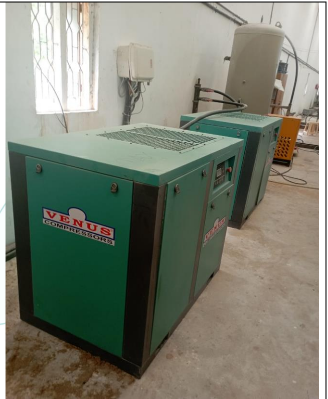
Air Compressor & Receiver Tank
