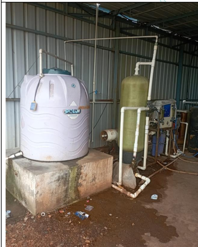
2000 LPH Water RO Plant
