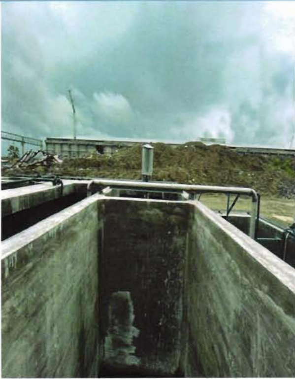
View of STP
