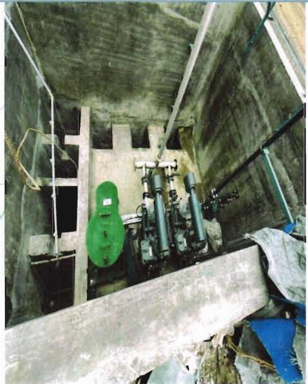
View of STP
