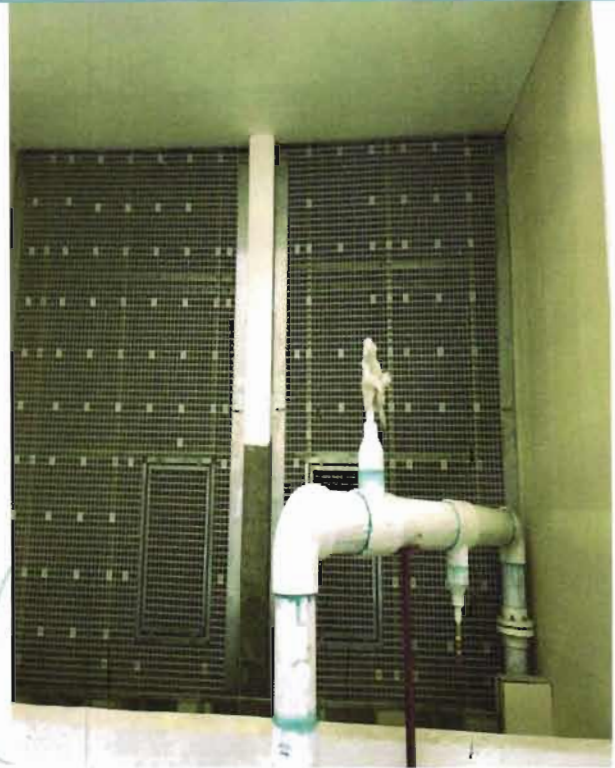
View of Luwa Humidification Plant
