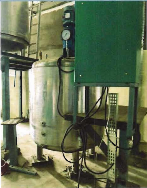
Tanks for Sizing Machine
