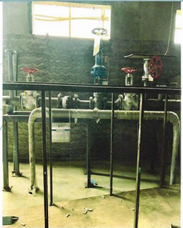
Forbes Marshall Pressure Reducing Station
