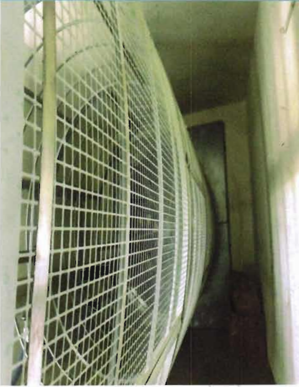
View of Luwa Humidification Plant
