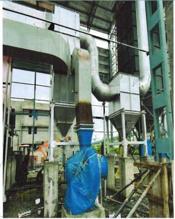
Dust Collection System
