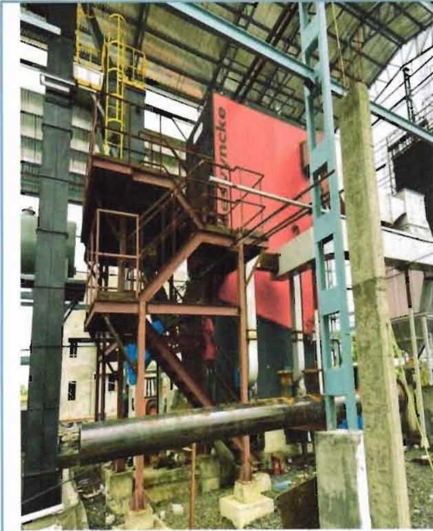
View of Boiler
