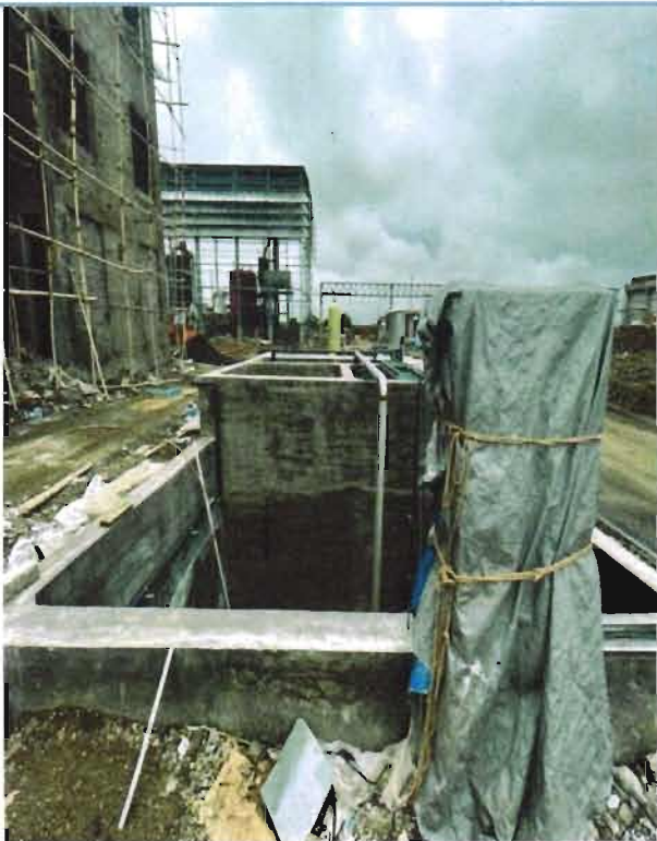
View of STP
