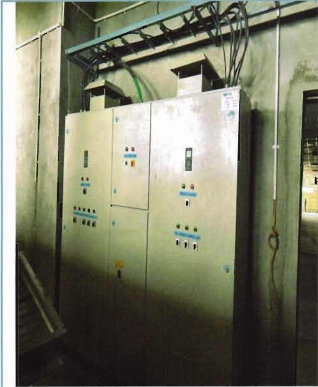
Panel for Humidification
