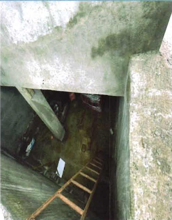
Fire Hydrant Pump Room
