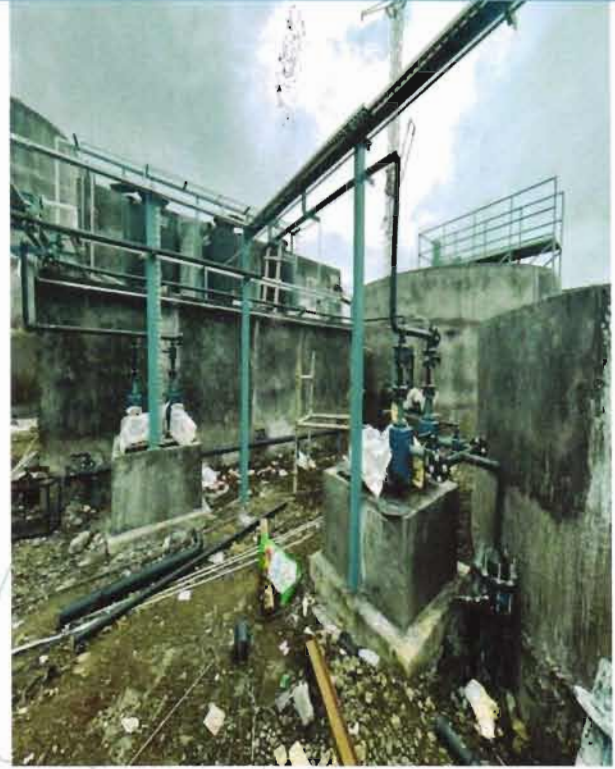
View of ETP
