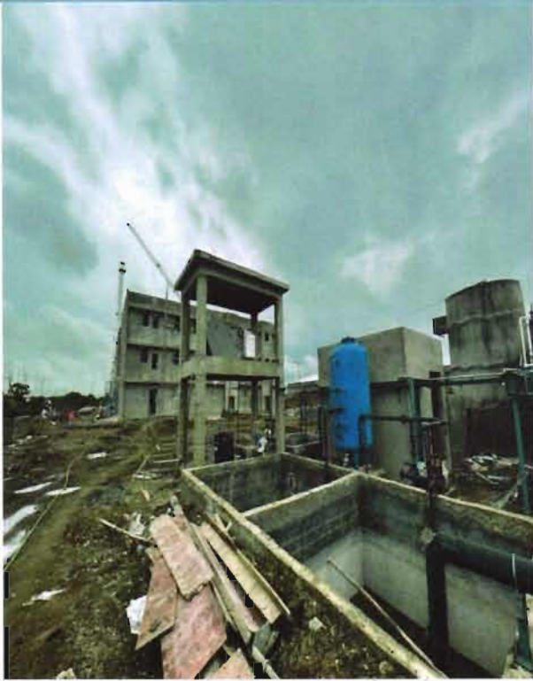
View of ETP
