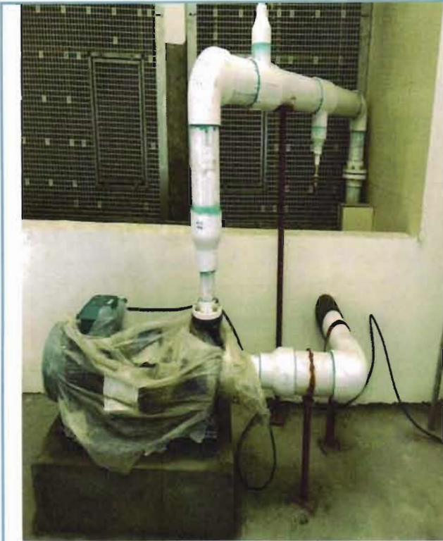
View of Luwa Humidification Plant
