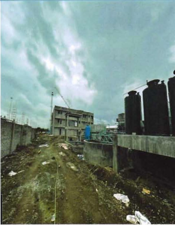
View of ETP
