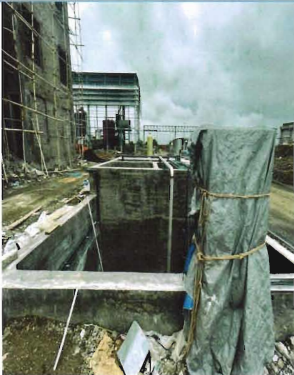
View of STP
