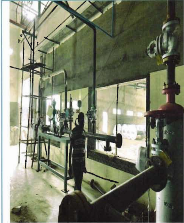
Forbes Marshall Pressure Reducing Station
