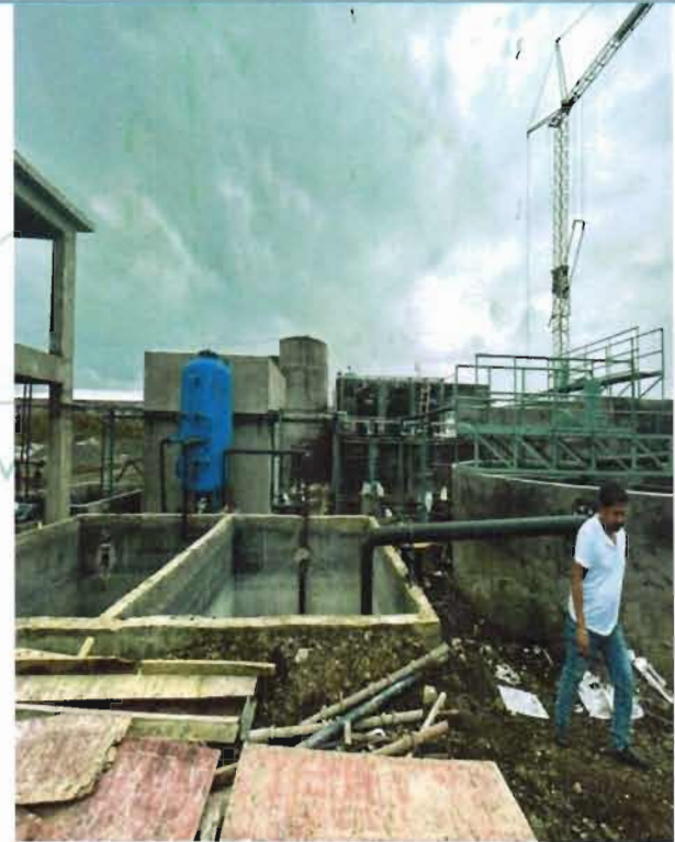
View of ETP
