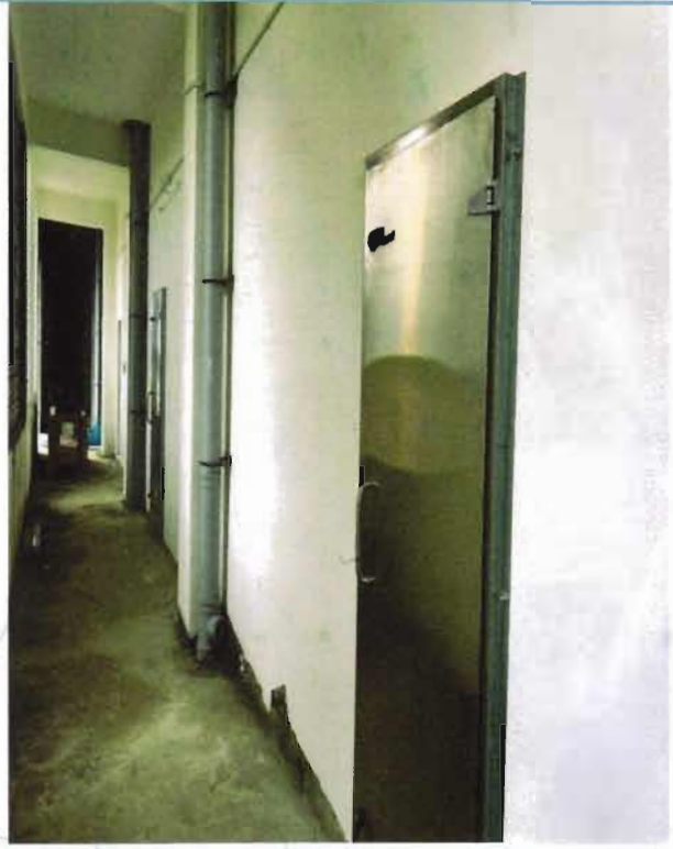
View of Luwa Humidification Plant
