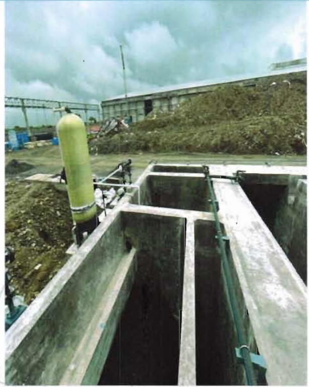
View of STP
