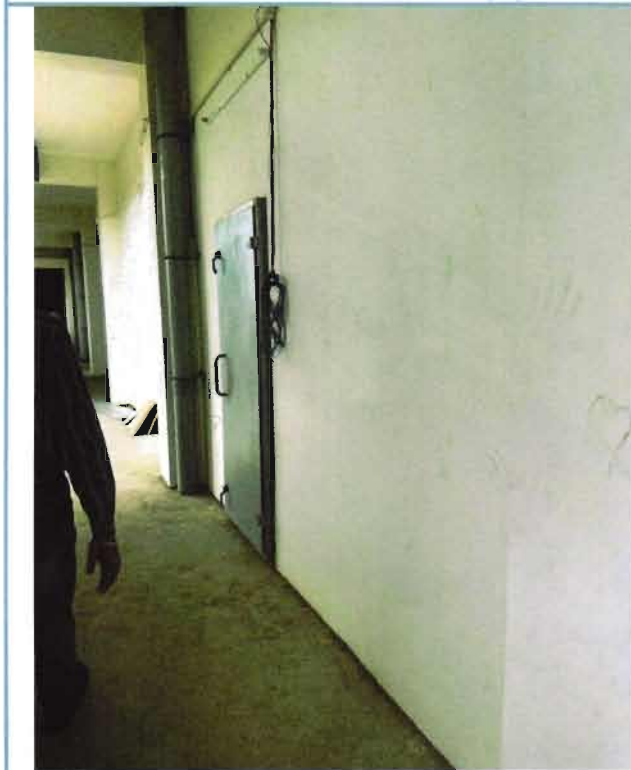
View of Luwa Humidification Plant
