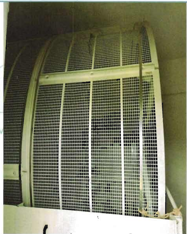
View of Luwa Humidification Plant
