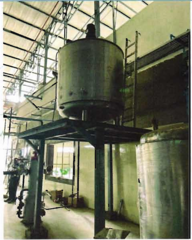
Tanks for Sizing Machine
