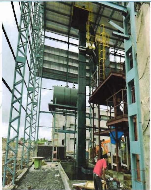
Fuel Feeding Conveyor
