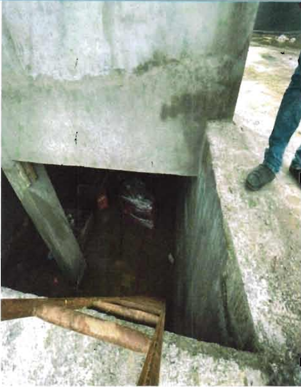
Fire Hydrant Pump Room
