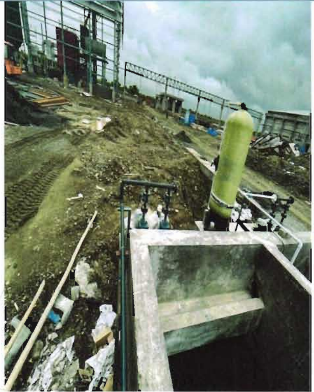
View of STP
