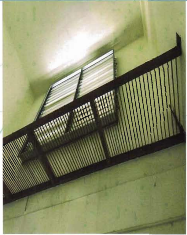
View of Luwa Humidification Plant
