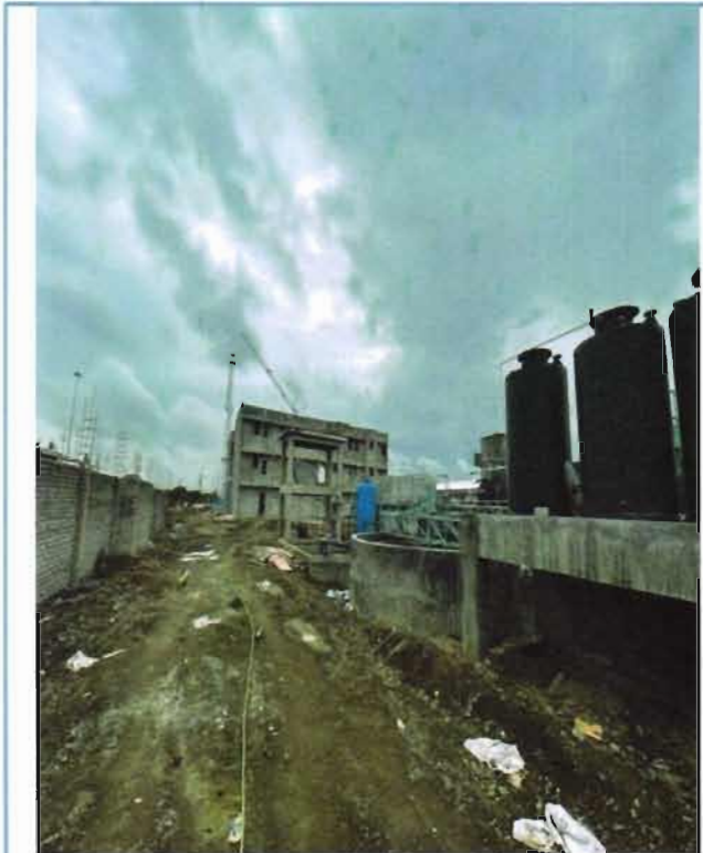
View of ETP
