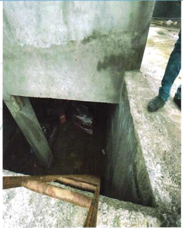
Fire Hydrant Pump Room
