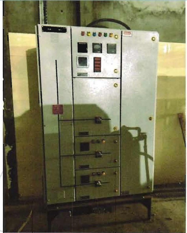
PDB-4 Electrical Panel for Warping
