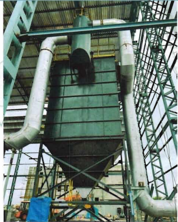
Dust Collection System
