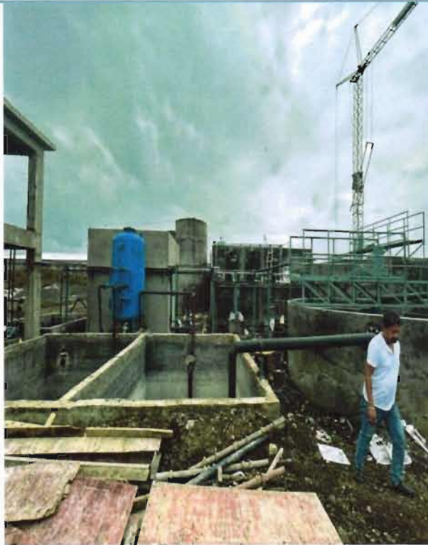
View of ETP
