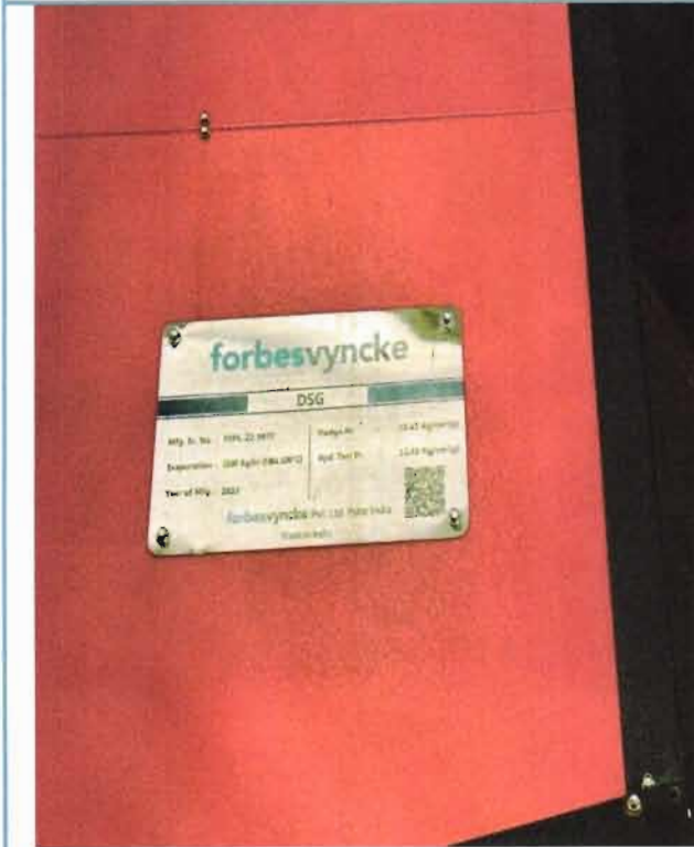
Boiler Name Plate
