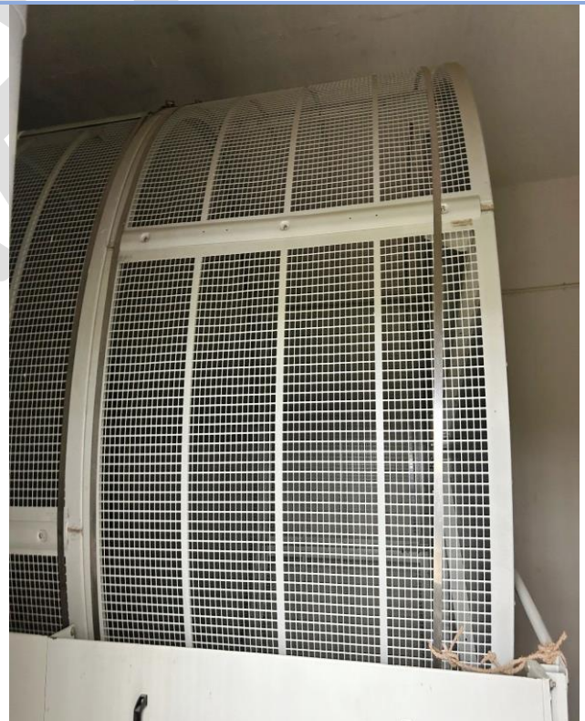
View of Luwa Humidification Plant
