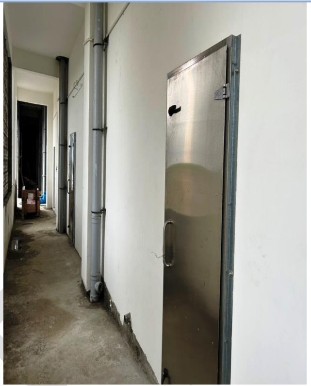
View of Luwa Humidification Plant
