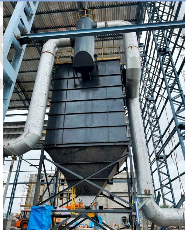
Dust Collection System
