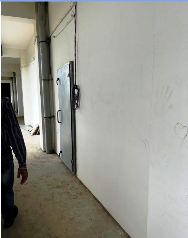
View of Luwa Humidification Plant
