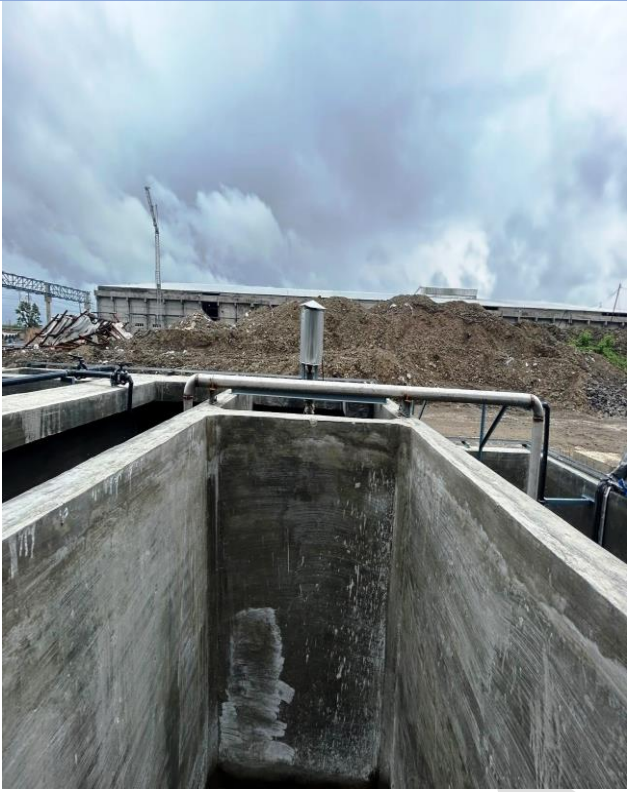
View of STP
