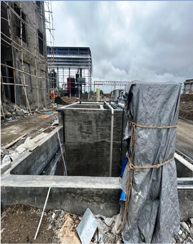
View of STP
