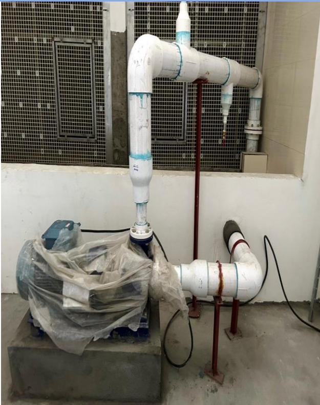
View of Luwa Humidification Plant
