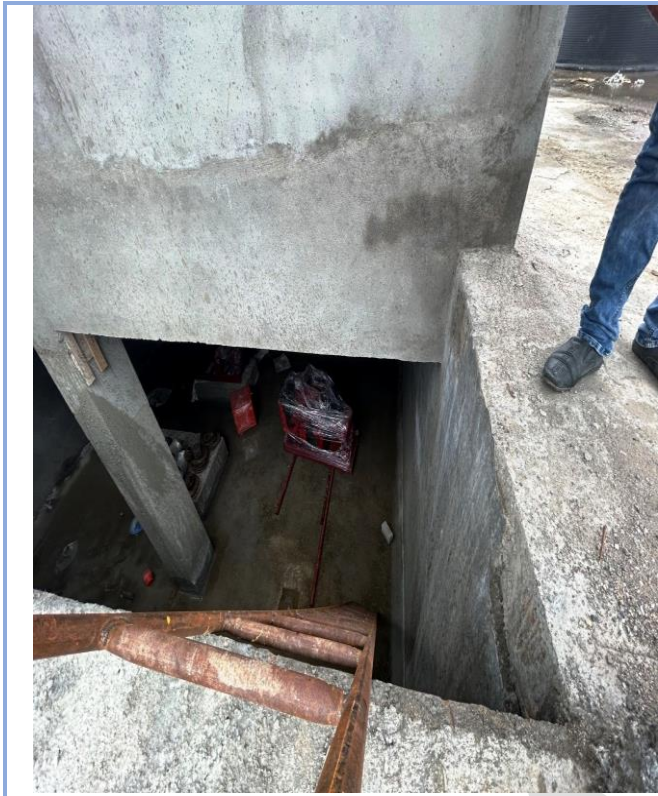
Fire Hydrant Pump Room
