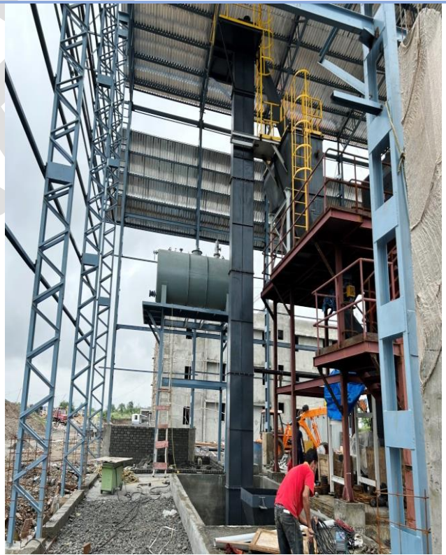
Fuel Feeding Conveyor
