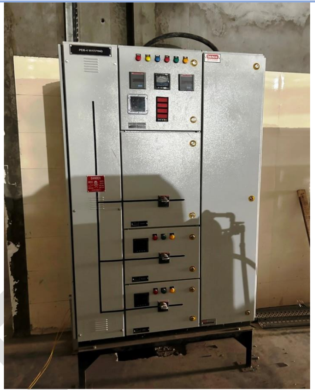
PDB-4 Electrical Panel for Warping
