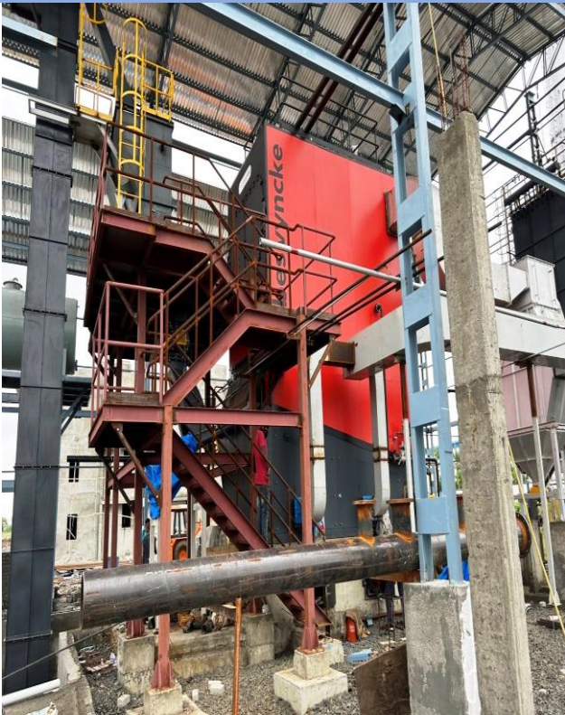
View of Boiler
