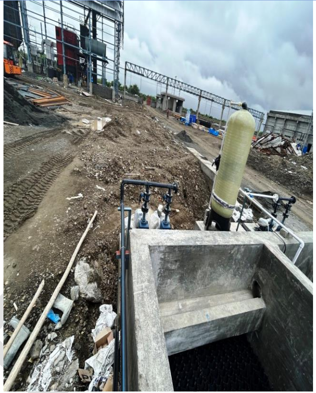
View of STP
