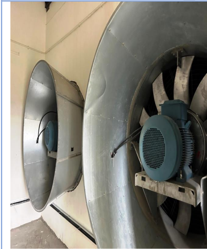
View of Luwa Humidification Plant
