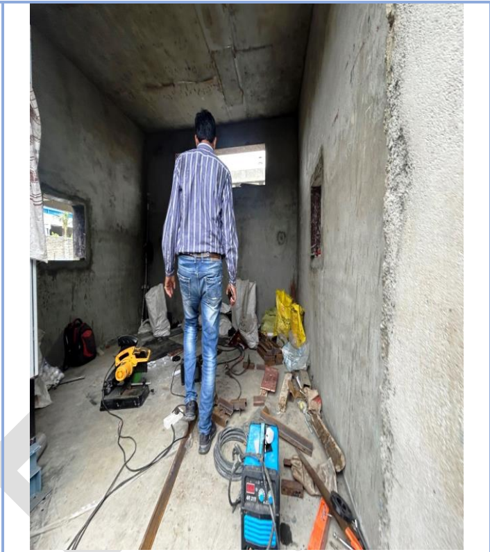
ETP Panel Room
