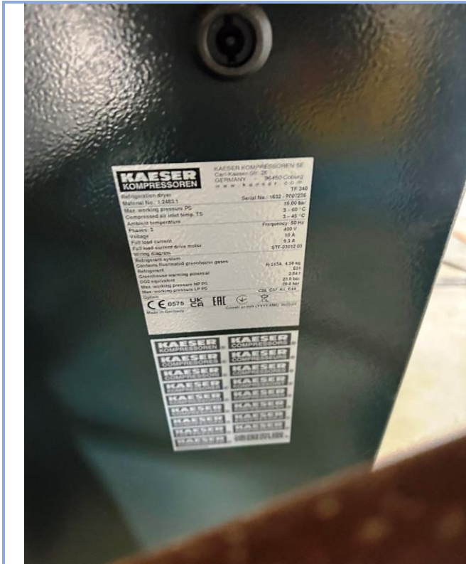
Name Plate of Refrigeration, (Sr. No. 1631)
