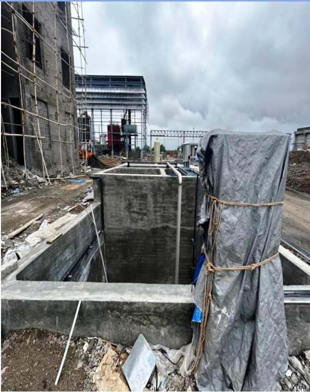
View of STP
