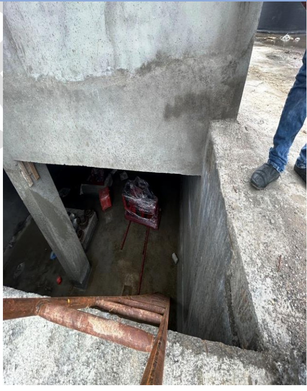
Fire Hydrant Pump Room
