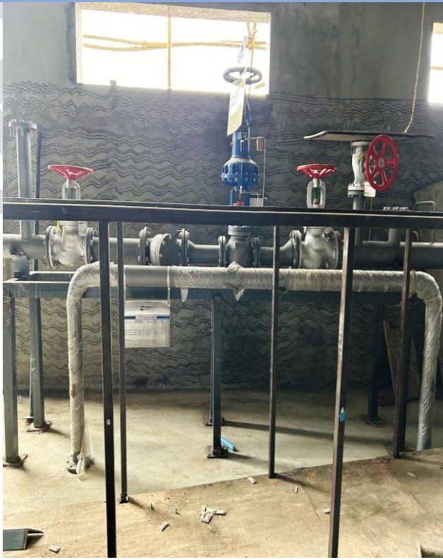
Forbes Marshall Pressure Reducing Station
