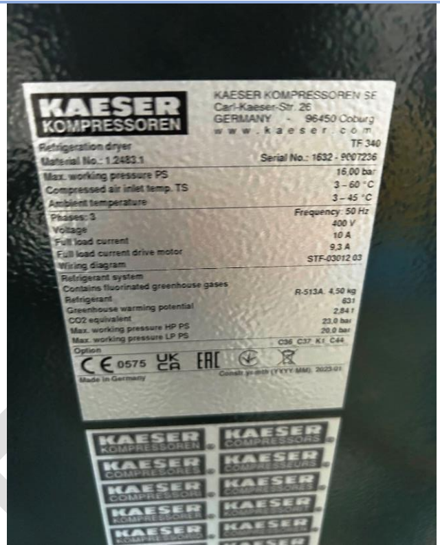
Name Plate of Refrigeration, (Sr. No. 1632)
