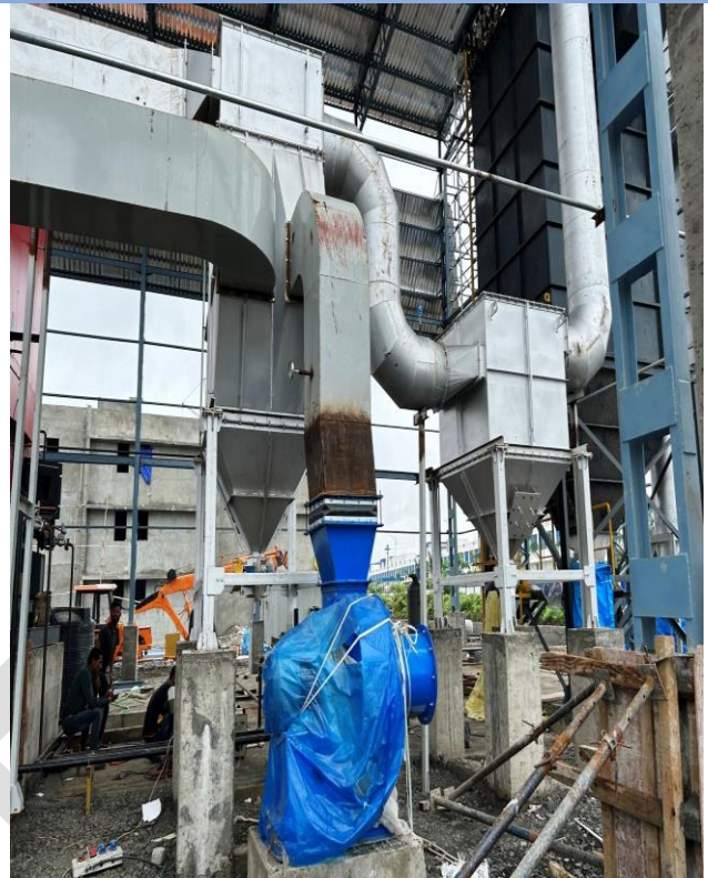
Dust Collection System
