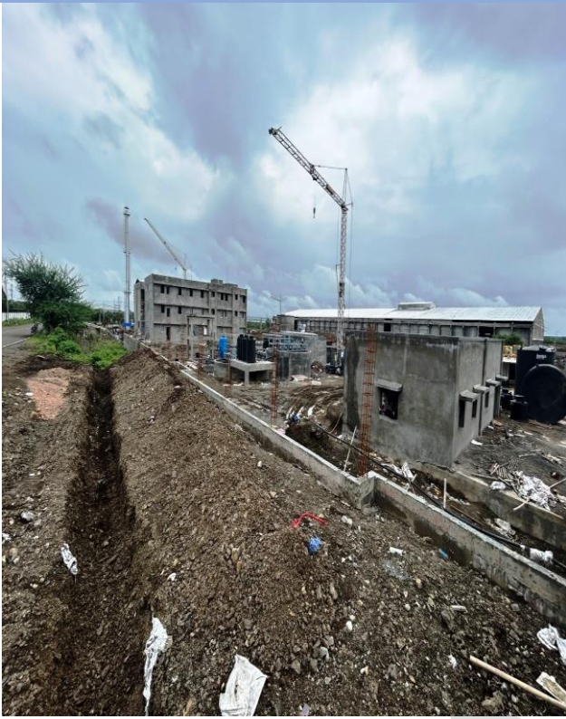
Storm Water Drain
