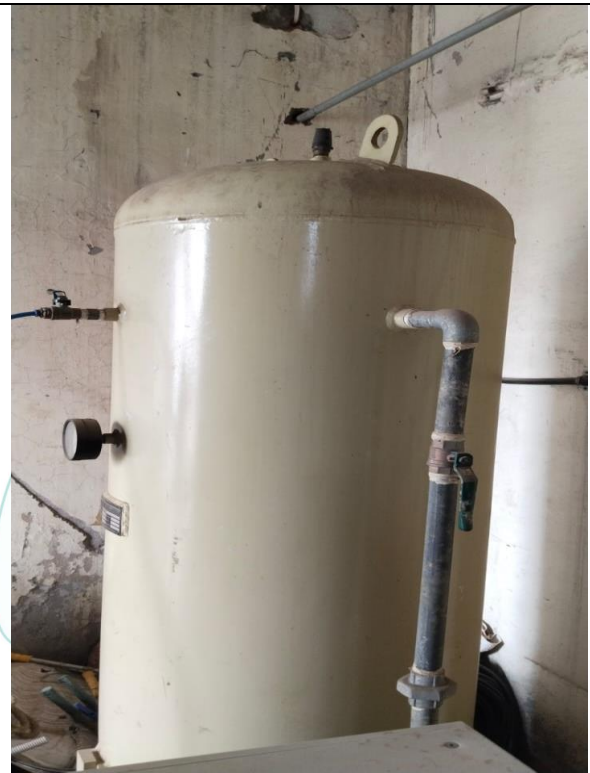
Air Receiver at Gurgaon Site-2
