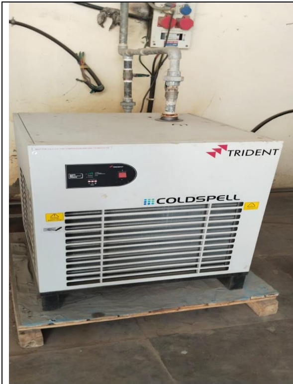
Air Dryer at Gurgaon Site-2
