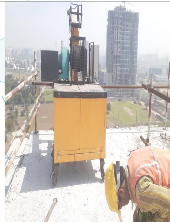
Floor Crane at Gurgaon Site-1
