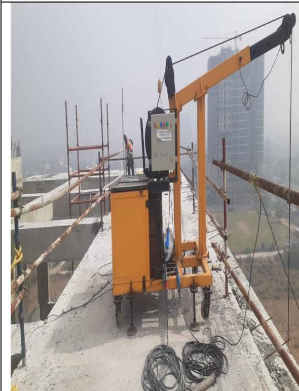
Floor Crane at Gurgaon Site-1
