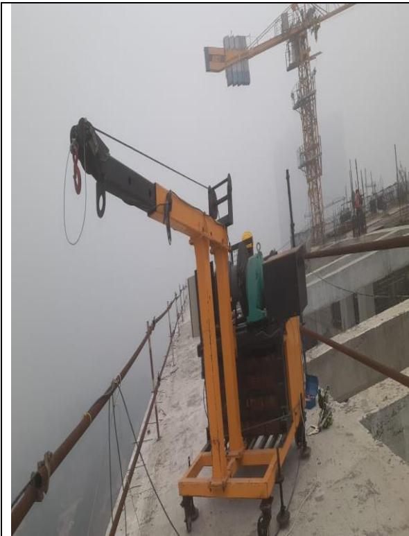
Floor Crane at Gurgaon Site-1
