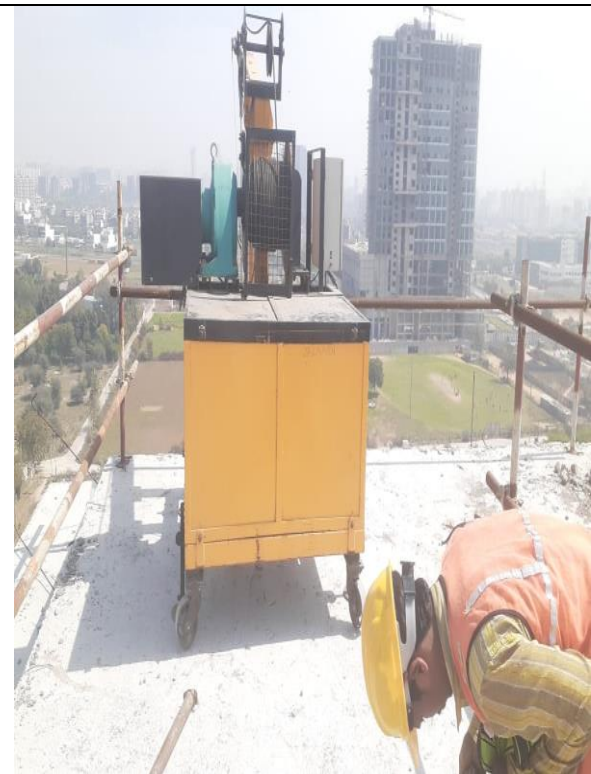
Floor Crane at Gurgaon Site-1
