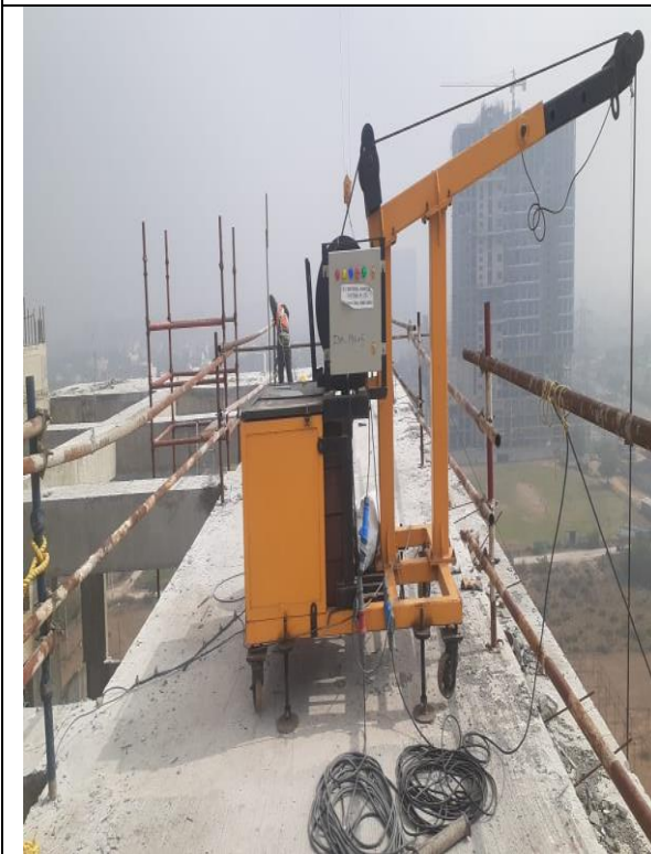
Floor Crane at Gurgaon Site-1
