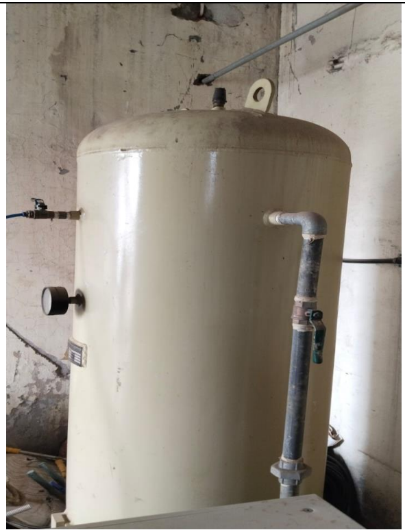
Air Receiver at Gurgaon Site-2
