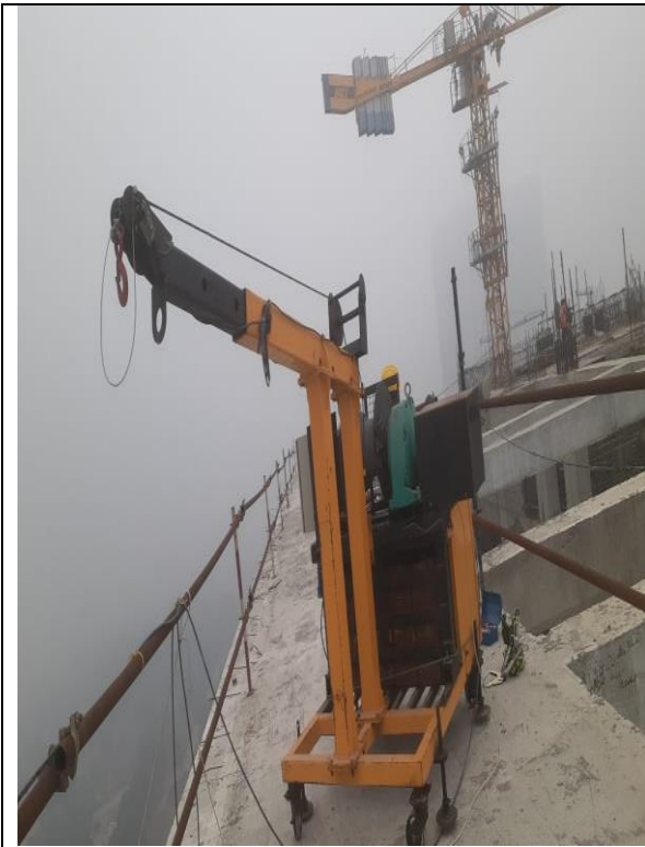
Floor Crane at Gurgaon Site-1
