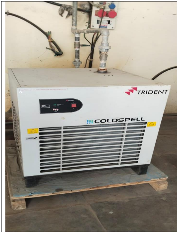
Air Dryer at Gurgaon Site-2
