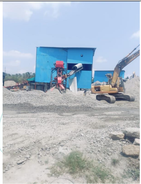
View of Stone Crusher Plant
